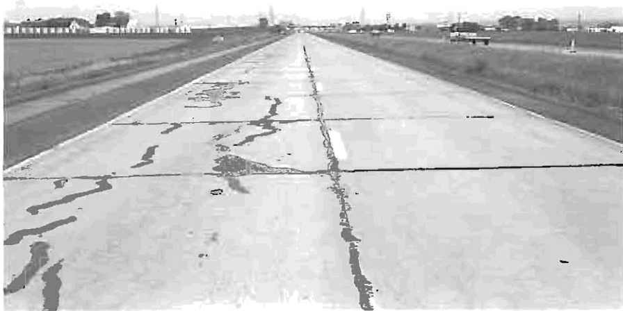
Photo 1 - Eastbound lanes I-76 between MP 13.87 and MP 16.37. Five foot of the outside shoulder was planned \frac{3}{4} of an inch and four foot of the inside shoulder was planned.
