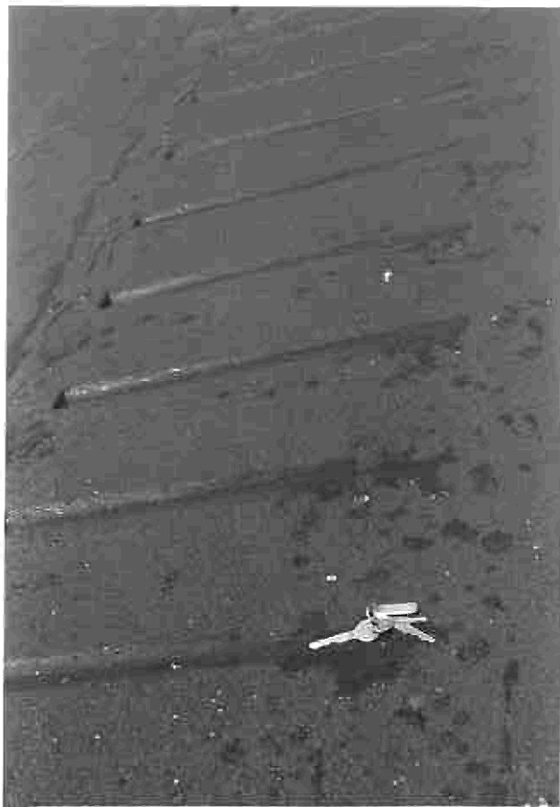
Photo 14 - Rumble strip without proper depth due to low asphalt temperature during placement.
