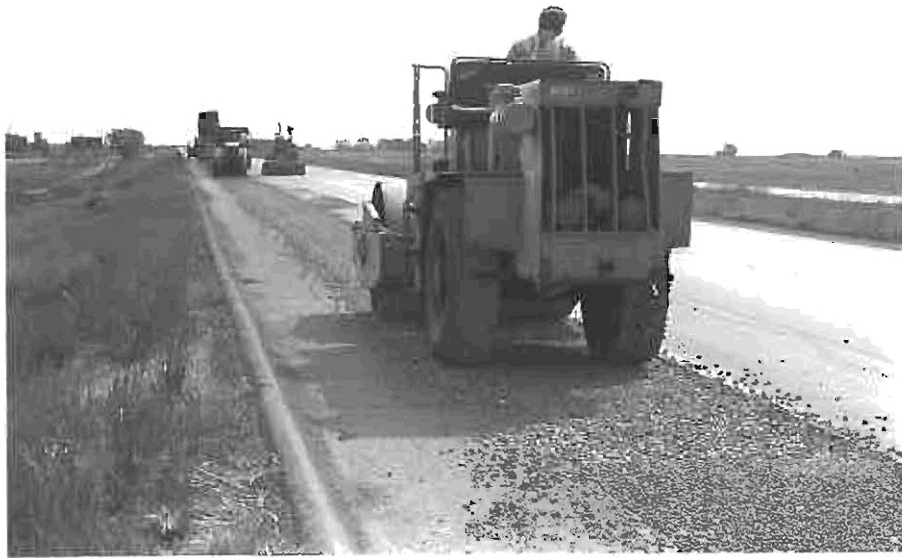
Photo 7 - The chips were rolled into the emulsified asphalt first by a rubber tired roller and then followed by a lite weight steel roller.
