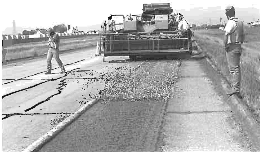
Photo 6 - Five feet of the outside shoulder was left uncovered by the chip seal for bike traffic.
