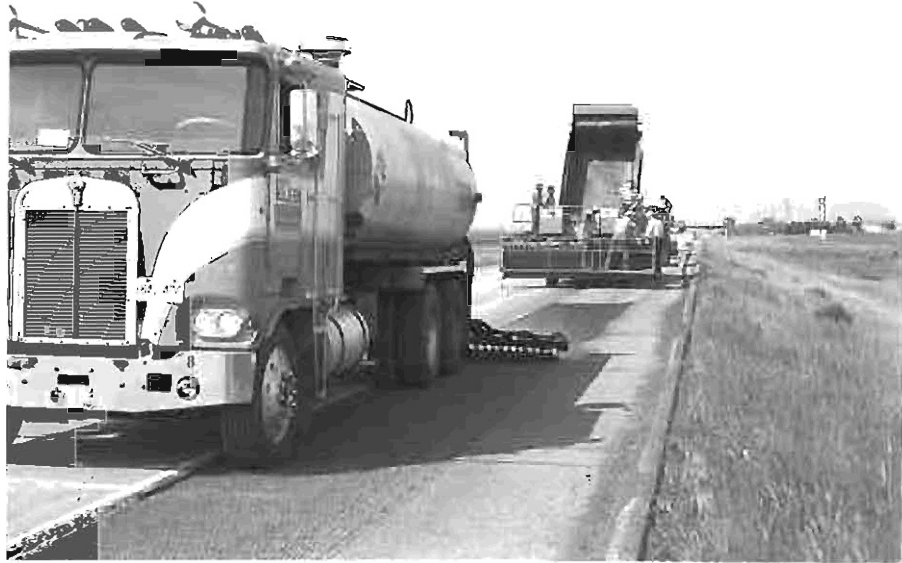
Photo 3 - Emulsified asphalt was rapid-setting, polymerized placed at 0.9 gallons per square yard. Original plans called for 0.4 gallons per square yard.
