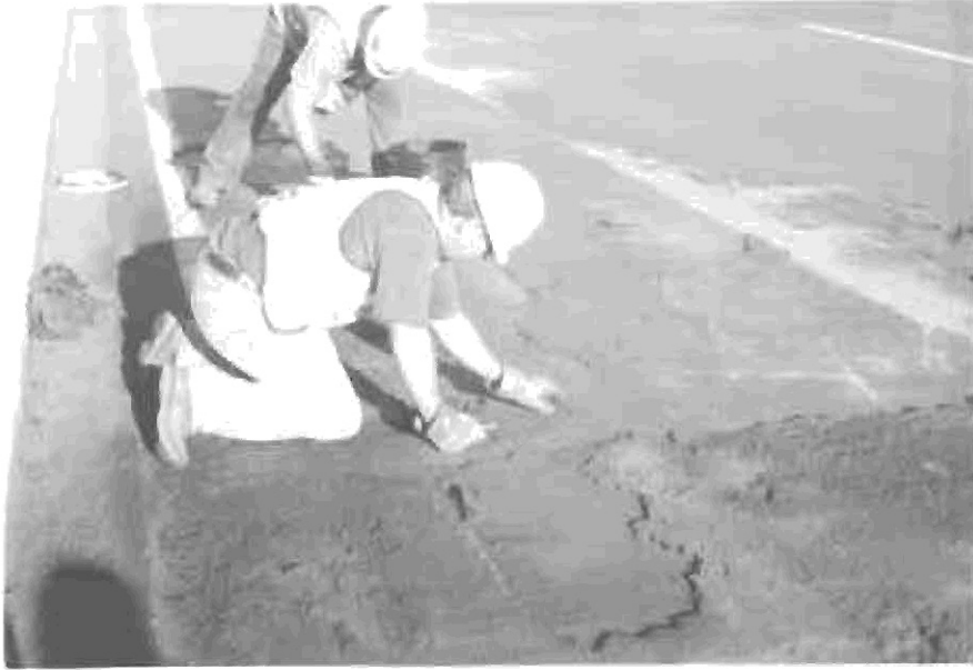
Figure 5. The exposed membrane was removed.
