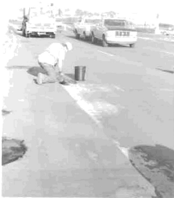
Figure 6. A cold-pour material was used to cover the area where the membrane was removed.
