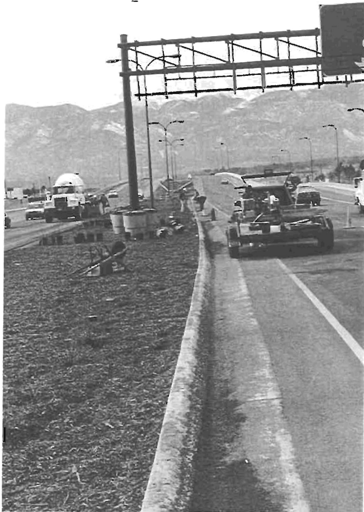
Type 2 curb and gutter meets type K1 keyed curb just beyond the sign post
