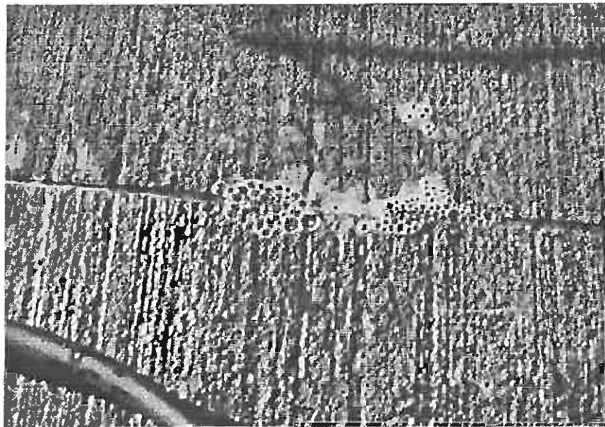
Figure 8 Bubbles show a leak in the seal. The larger bubbles to the left indicate a larger leak than the one to the right. The small bubbles to the rear of the joint may indicate a pinhole in the concrete or a micro crack that could develop into a spall.
