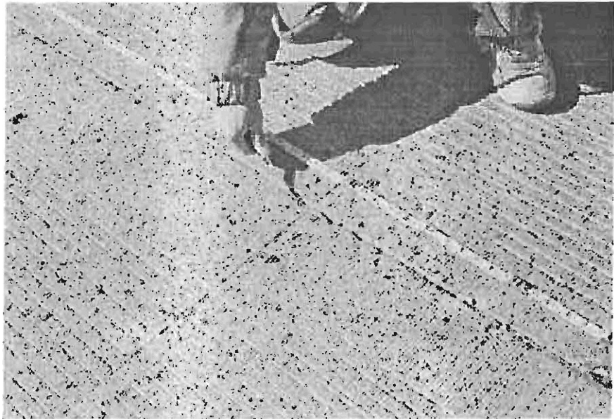
Figure 11 During a visual inspection of new seals, the only way to check for adhesion of the seal to the walls of the joint is to probe the seal and watch for it to move away from the wall. It is also necessary to probe spalls to see if they extend below the seal.
