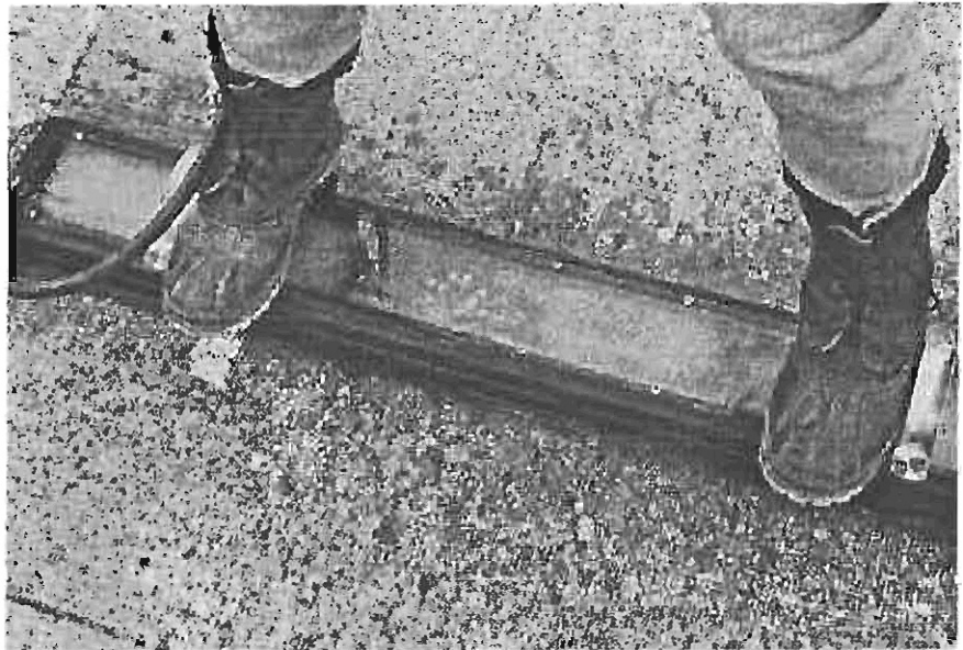
Figure 9 The drops on the glass show a large failure that is passing air too rapidly for bubbles to form. A failure this large is usually easily seen.
