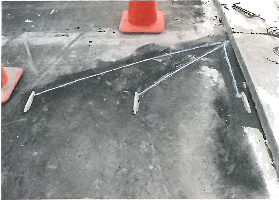
Figure A.5 - Asphalt Surface and Concrete Embedment Gages Prior to Concrete Placement
