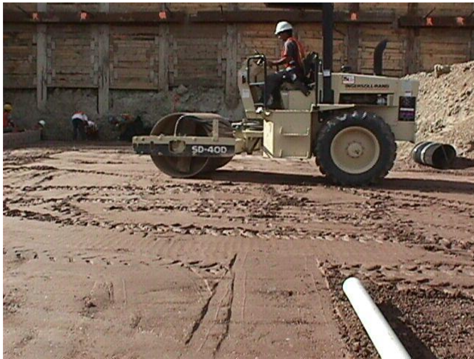
Figure B-21. A vibratory roller was used to compact the fill material.
