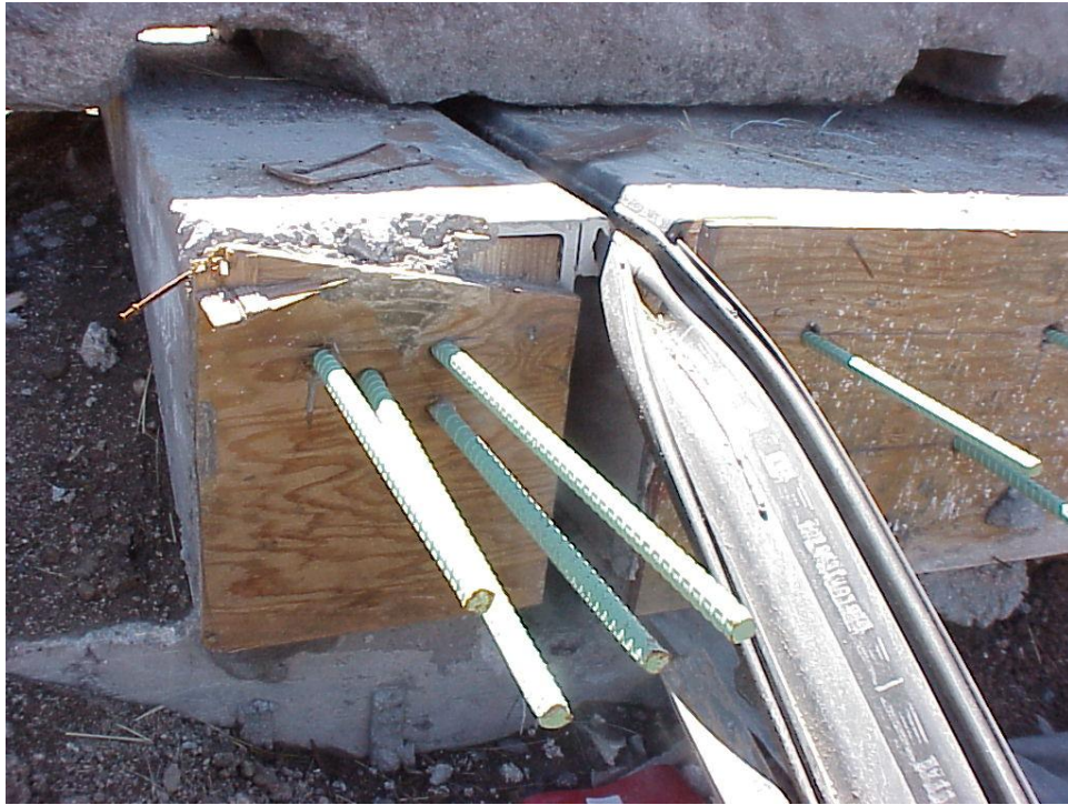
Figure B-43. The approach expansion device placed between the sleeper foundation and approach slab.
