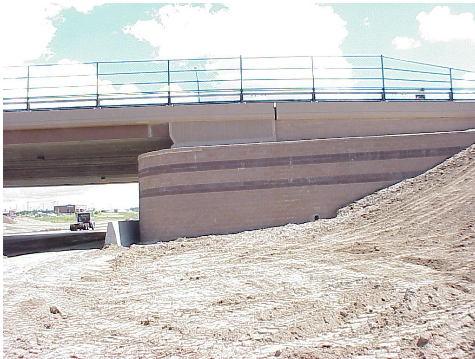
Figure B-1. A view of the northwest side of the completed Founders/Meadows bridge-approaching roadway structure showing lower and upper MSE walls, wing walls, and girders.
