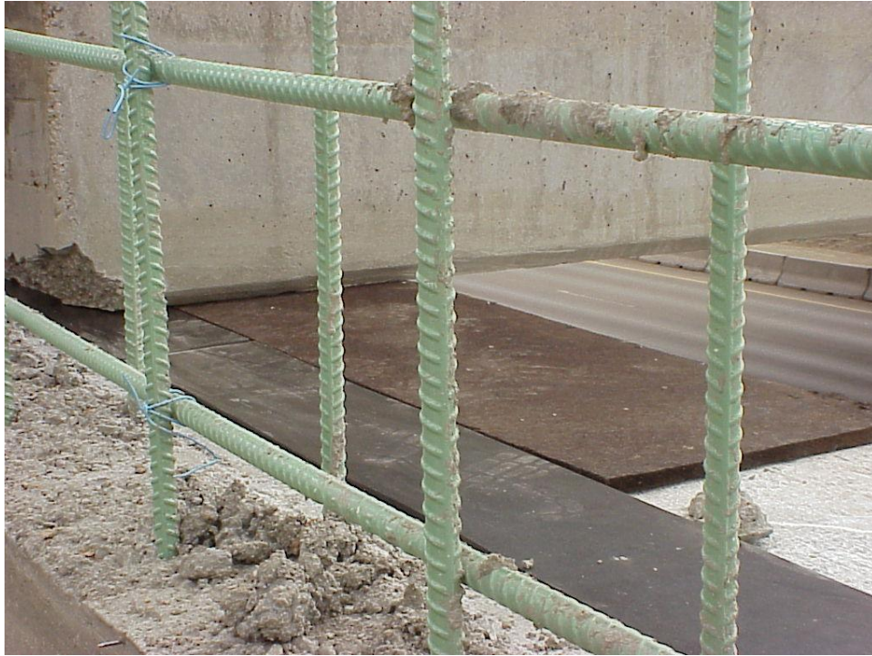
Figure B-31. The elastomeric bearing pad and expansion joints material placed on the abutment wall where girders will be seated.
