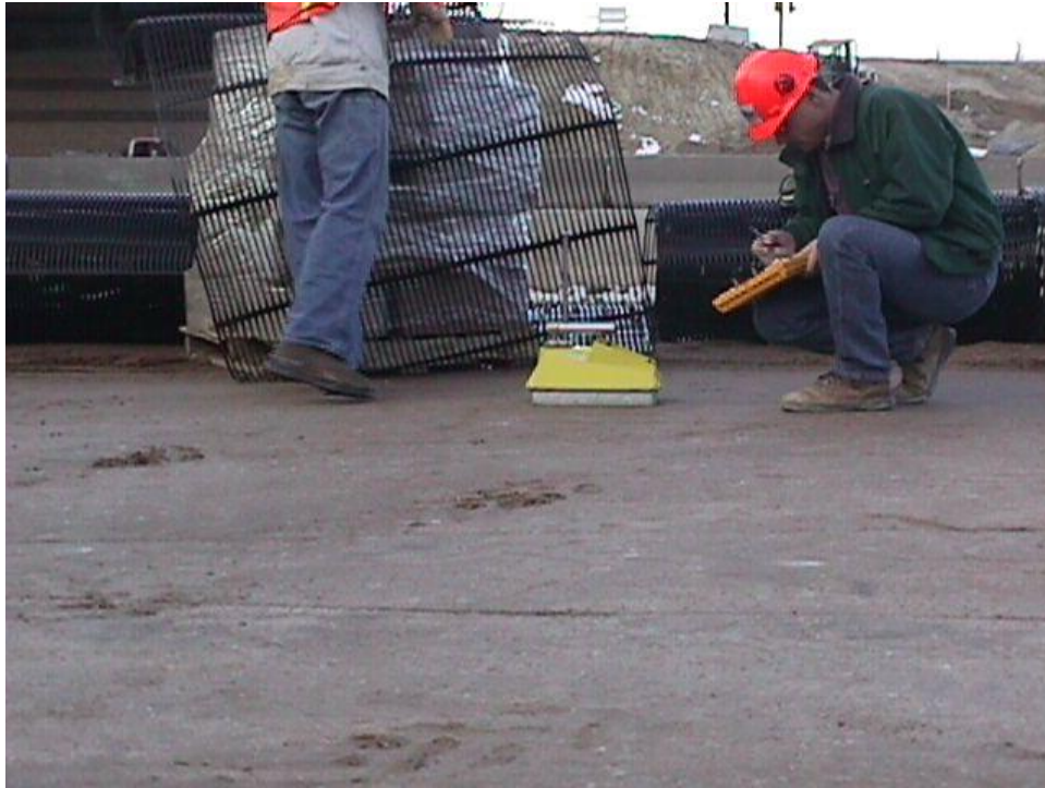
Figure B-15. Backfill levels of compaction were checked with a nuclear gage.
