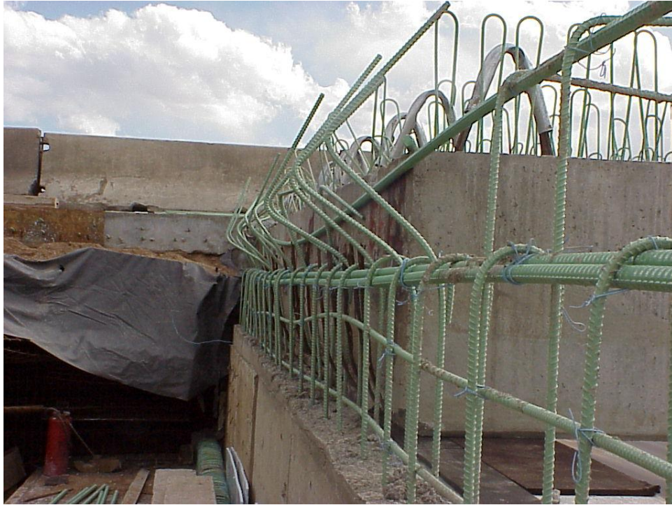
Figure B-33. Abutment wall and some girders. The stage that follows is pouring the concrete for the bridge deck and the rest of the abutment wall and girders. The overlapping steel from girders, abutment wall, and bridge deck will strongly attach the bridge superstructure to the abutment wall without any joint (integral abutment).
