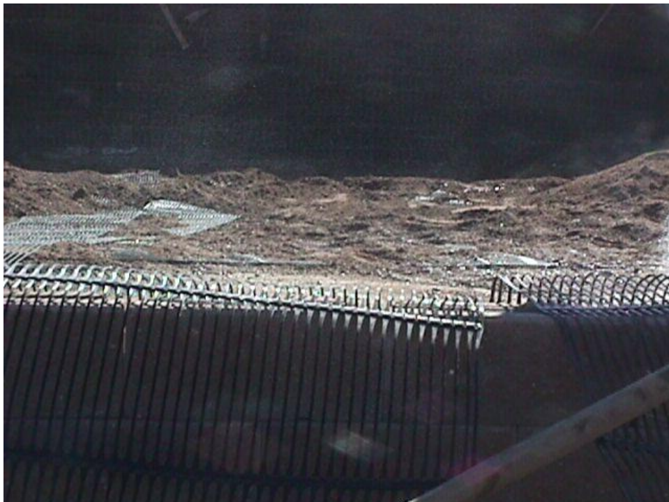
Figure B-16. Around the corners of the lower MSE walls, where geogrid from the front and side of the structure overlapped, a thin layer of fill material was placed between these geogrid layers to provide friction between them.
