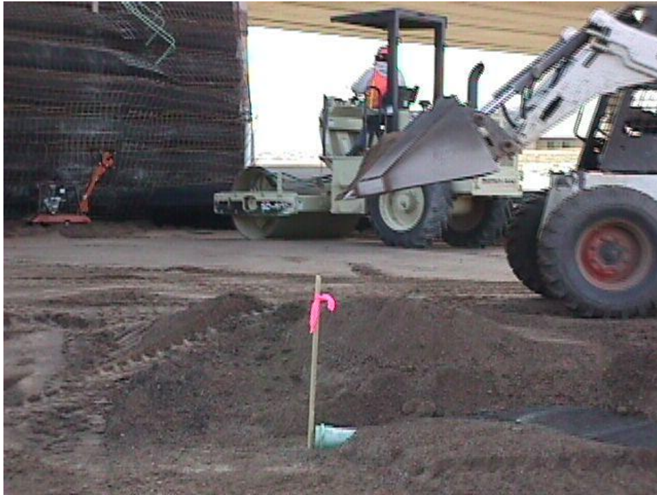
Figure B-25. The pipe used with the drainage blanket placed behind the reinforced backfill.
