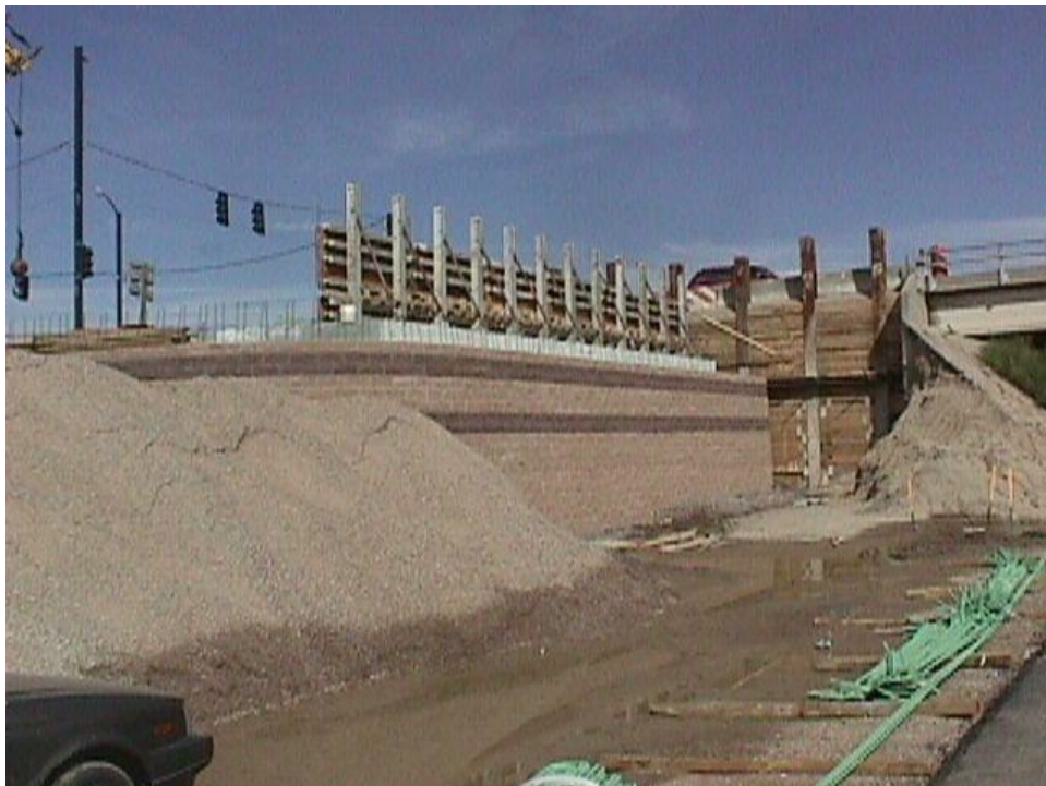
Figure B-26. The abutment wall footing has been poured and the forms are being set for the abutment wall.
