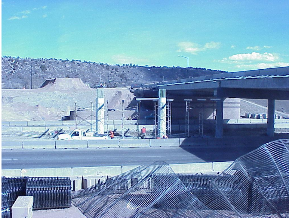
Figure B-7. Rolls of Tensar UX 6 geogrid placed below the bridge foundation.
