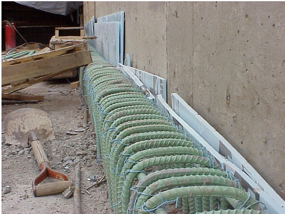
Figure B-32. A reinforced concrete “kicker” strongly attached to the bridge foundation was placed behind the bottom of the abutment wall. This kicker was placed to provide an extra bracing at the top of MSE wall for global stability.
