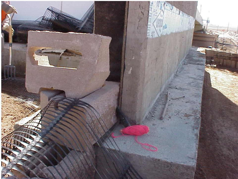
Figure B-38. The edge of the wing wall and upper MSE wall. Expansion joint material was placed between blocks and leveling pad and between blocks and the wing walls.
