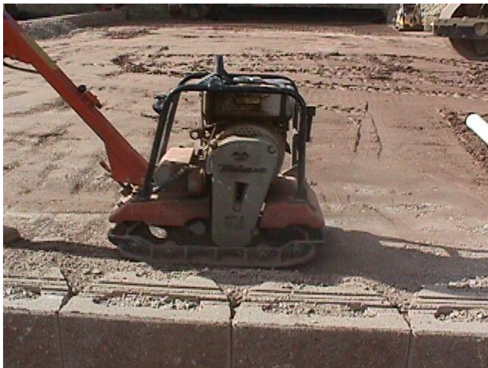
Figure B-22. Near the block facing, a small walk-behind compactor was used to prevent pushing the blocks out of position.
