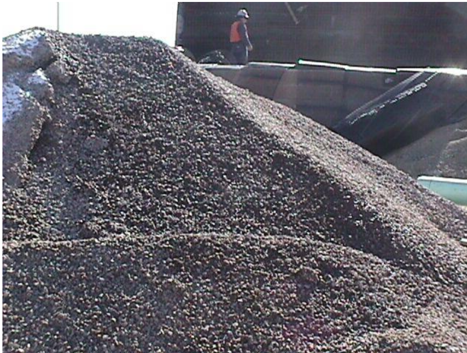
Figure B-6. The 19 mm maximum size crushed stone aggregate used to fill in and for .3 m behind the blocks to facilitate compaction and drainage behind the blocks, prevent washout of the fines in the fill material, and facilitate compaction behind the facing.
