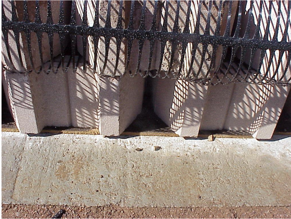
Figure B-13. Expansion joint material was placed between the leveling bed and the first row of blocks.
