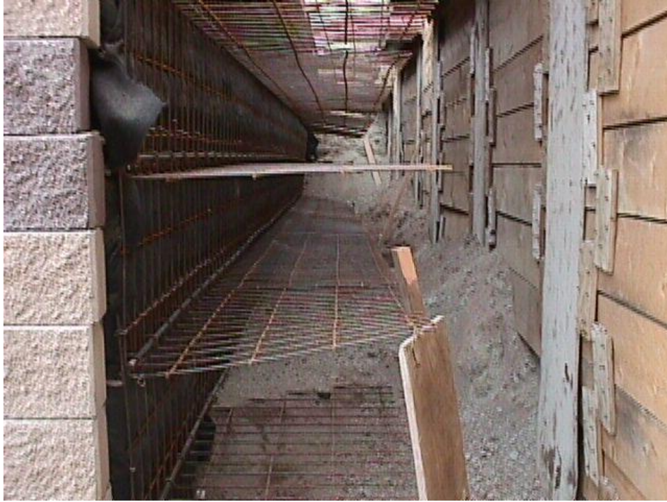
Figure B-19. Temporary wire mesh facing was used to support the northern face of the Phase I structure until the Phase II structure was built and tied to the Phase I structure. The backfill in between the wire mesh reinforcement was contained using wrapped fabric that also facilitated backfill drainage. To the right is a closer look at the shoring supporting the old bridge structure.
