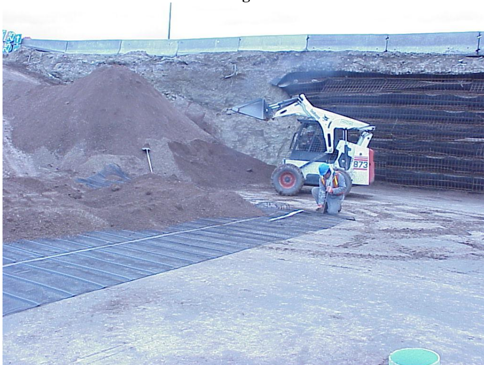
Figure B-20. The geogrid was connected at the wall end, rolled out, and then stretched by hand. The back end was staked to prevent geogrid movement while the fill was placed using a small loader. In the background is the steel reinforcement used to temporarily support the northern face of the Phase I structure.
