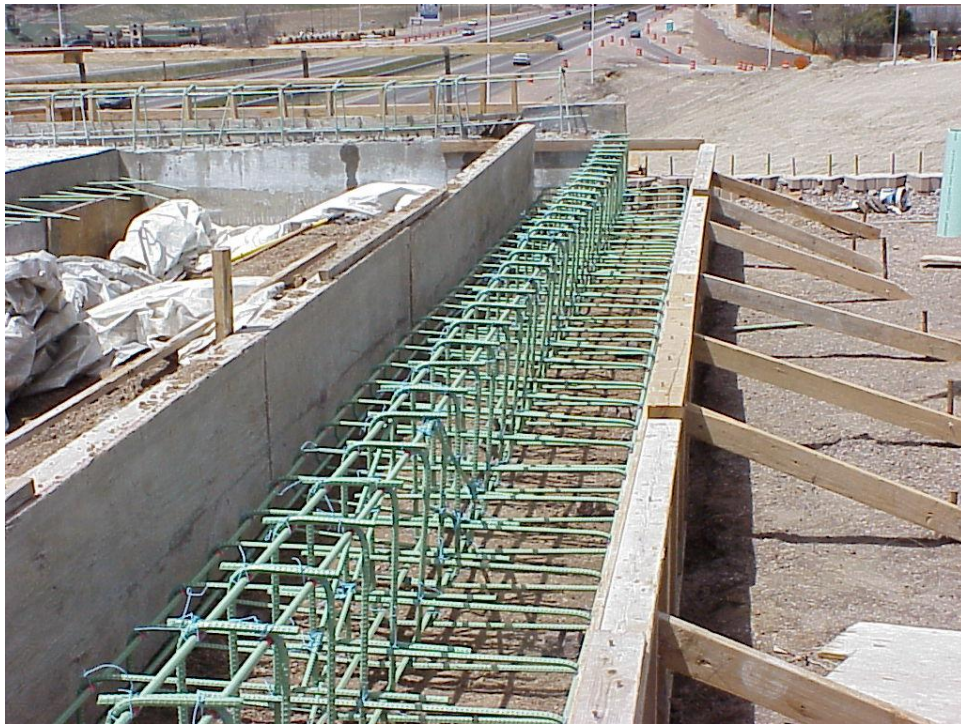
Figure B-42. The forms and reinforcing steel for the sleeper foundation supporting the approach slab.
