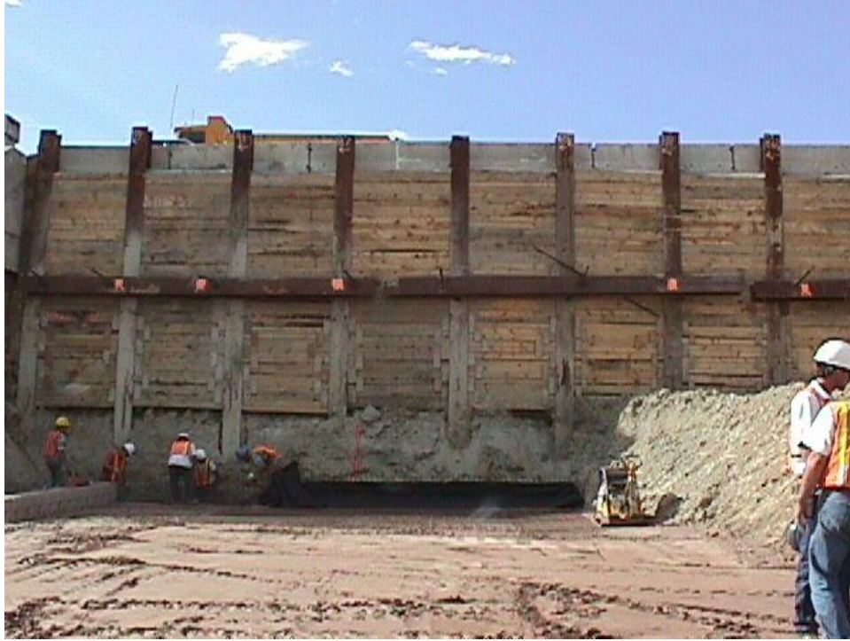
Figure B-17. The first layer of fill material at the east side of the Phase I Structure has been placed. In the background, H-beams and shoring support the approach to the old bridge during the construction of the Phase I Structure.
