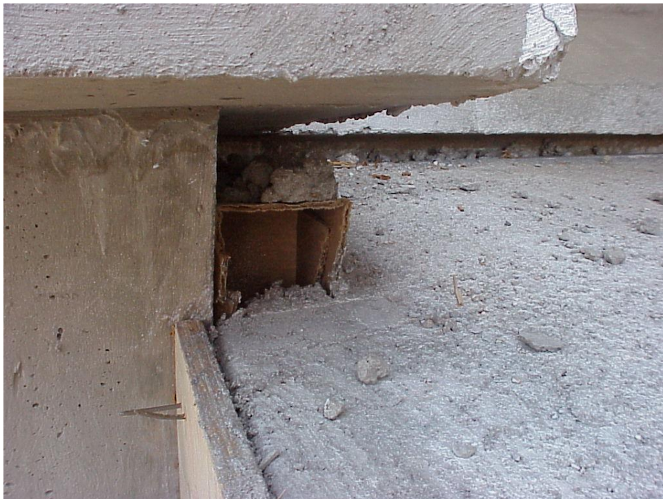
Figure B-40. Collapsible cardboard was placed in front of the bottom portion of the abutment wall behind slope paving (see figures 29 and 35).
