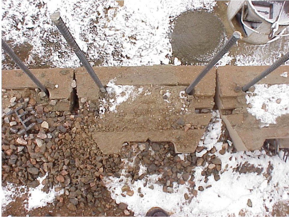
Figure B-27. The top two rows of blocks were filled with concrete. Steel rebars inserted in the plastic concrete were later bent over to tie the concrete cap at the top of the front MSE wall.
