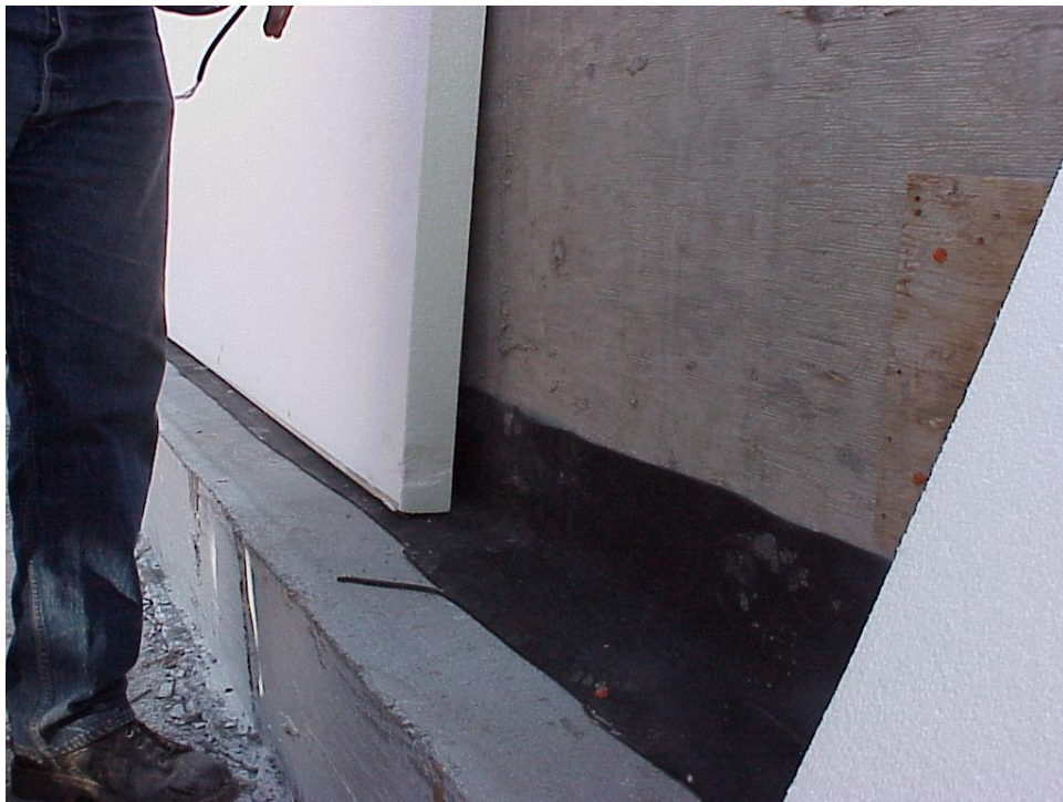
Figure B-34. A plastic sheet was placed between bridge abutment and bridge foundation to facilitate water drainage.
