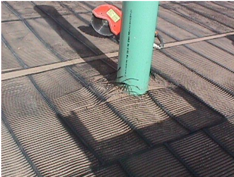
Figure B-24. The geogrid was cut to fit over a drain pipe that went down through the middle of the structure. The pieces of geogrid were offset from one layer to the next so the longitudinal joints did not line up vertically.
