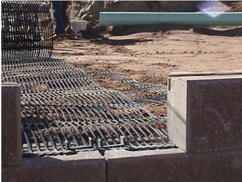
Figure B-11. The facing blocks are fastened to the geogrid by the use of Mesa Standard Connectors which fit into the grooves of the blocks.
