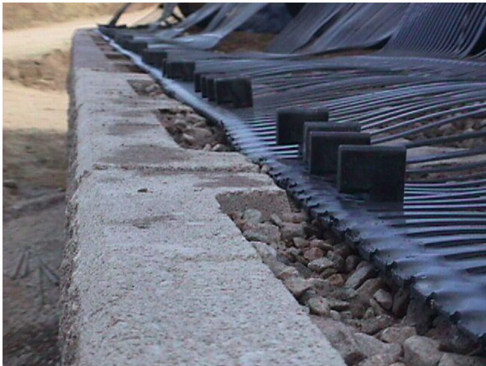
Figure B-12. The rear of the block (to the right of the picture under the geogrid) is lower than than the front to allow for the thickness of the grid.
