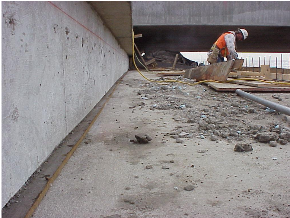
Figure B-28. Expansion joint material was installed below the sides of the abutment wall on top of the footing. In the center zone below the abutment wall on top of the footing, galvanized sheet metal centered on a bearing pad was placed (see figure 29).
