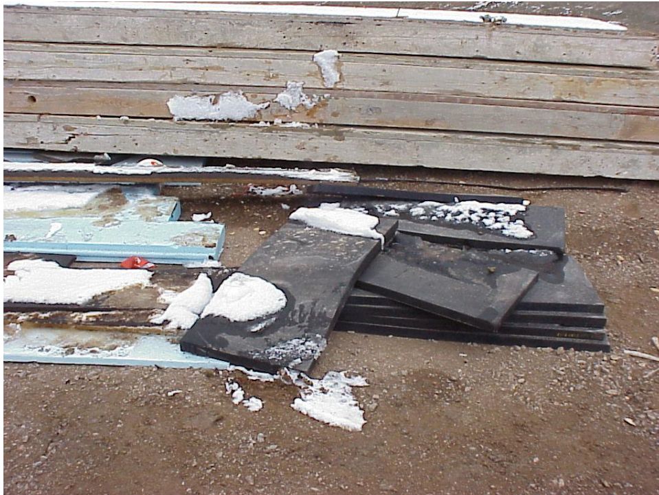
Figure B-30. These elastomeric bearing pads were installed on the abutment wall where the bridge girders are seated.
