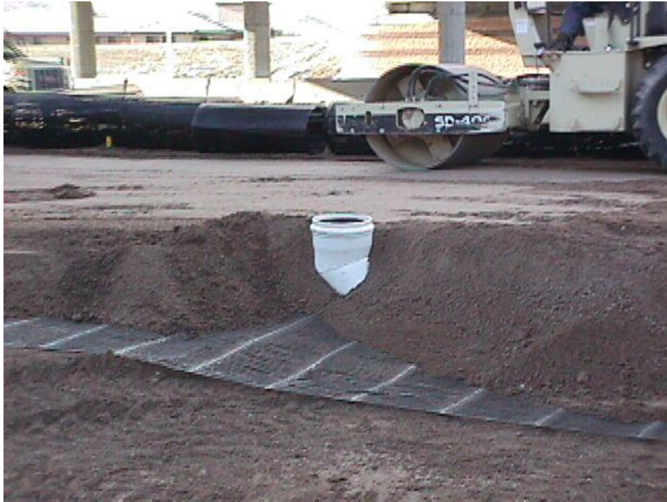
Figure B-23. A vertical drain pipe was installed inside the MSE Walls.
