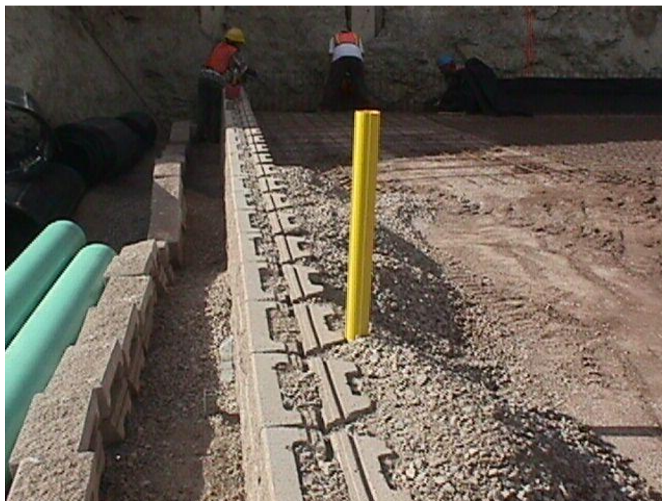
Figure B-4. Picture showing facing blocks, crushed stone used to fill in and 0.3 m behind the blocks, and the compacted CDOT Class 1 backfill. The yellow inclinometer tube was used to measure lateral movement in the structure along Section 400.
