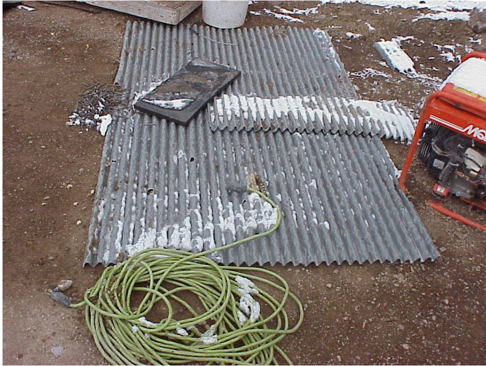
Figure B-39. This panel was used to give texture to the outside of surface of the concrete wing wall.
