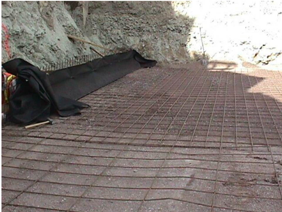
Figure B-18. The northern side of Phase I structure was internally stabilized with steel wire mesh. The steel extended past the edge of the wall and was tied to the geogrid placed to stabilize the front MSE wall.
