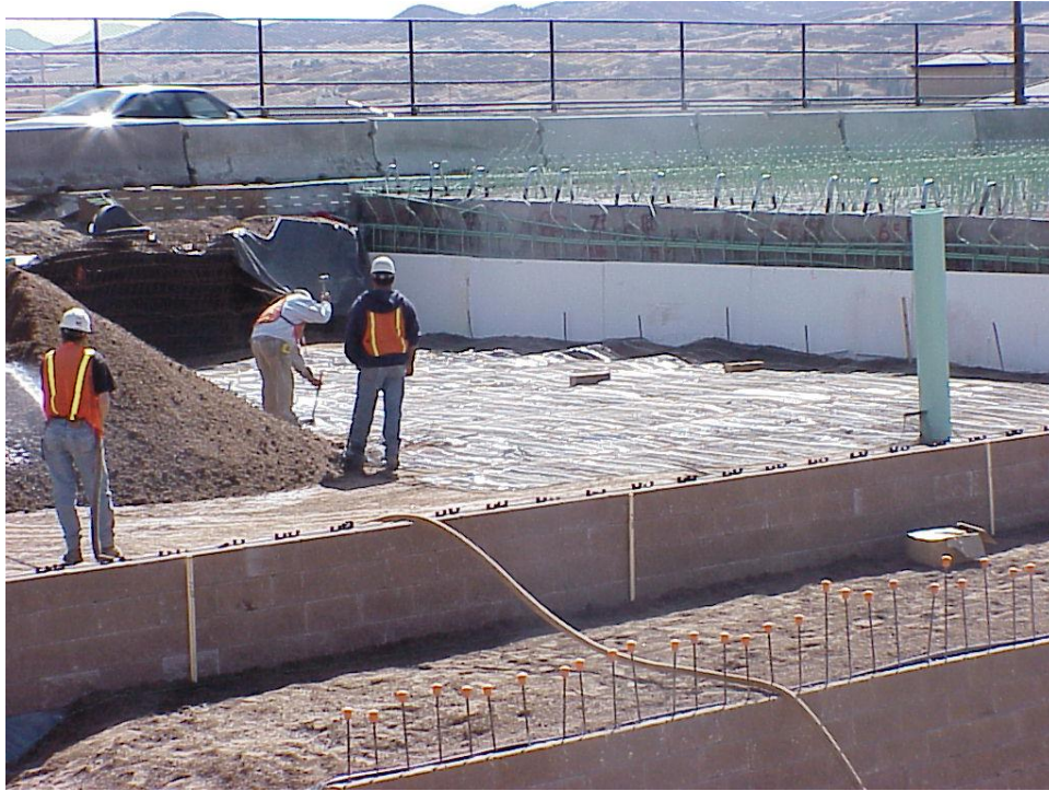
Figure B-35. After the girders were placed, 75 mm sheets of low-density expanded polystyrene were placed against the back of the abutment wall. The area in the foreground between the lower and upper MSE walls will be covered with a membrane and paved with concrete (referred to as slope paving in Fig. 40).
