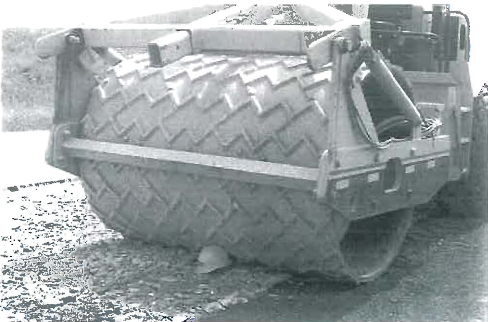
Figure 12. Steel vibratory roller with “Z” pattern grid on drum face was used to seat pavement.
