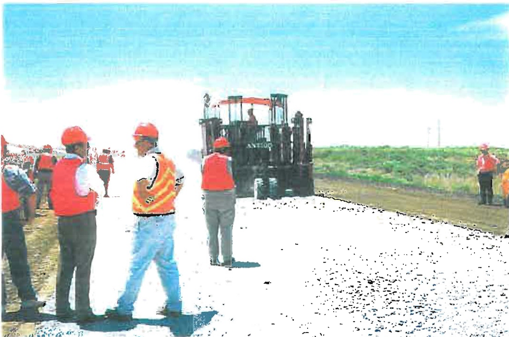
Figure 3. Field trip to project site enabled participants to observe the rubblization and crack & seat processes.
