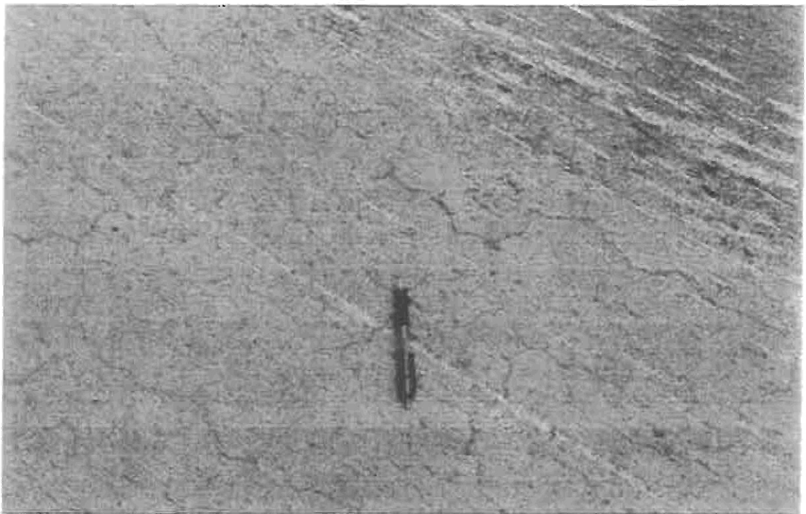
Figure 6. Photo shows the ASR distress found in the concrete pavement.
