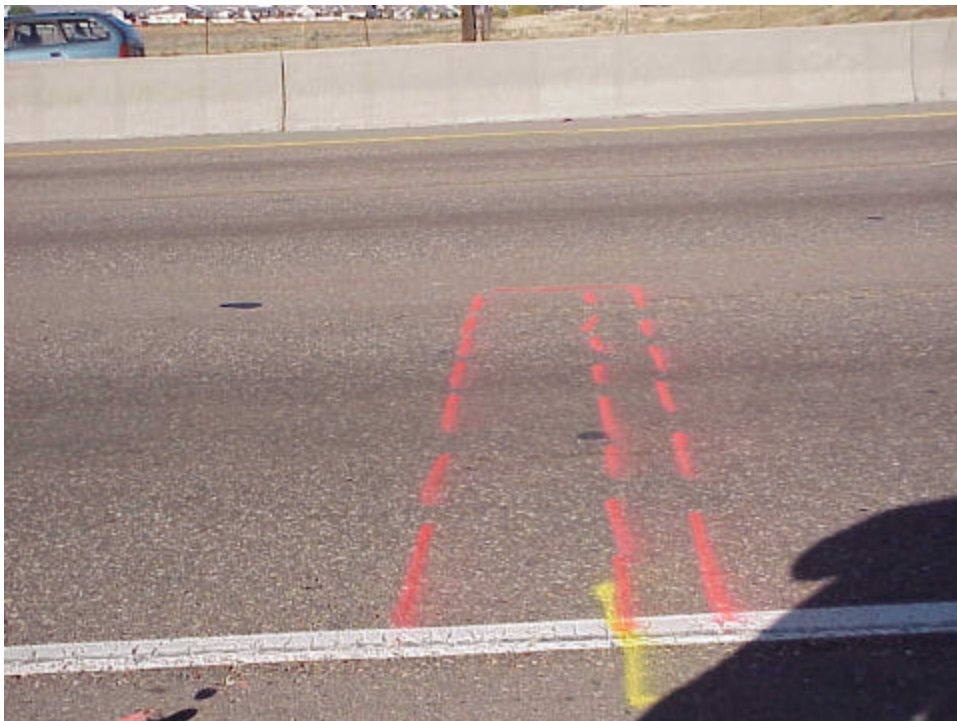
Location of the cross section slab before sawing. From this angle the longitudinal cracks are not readily visible.
