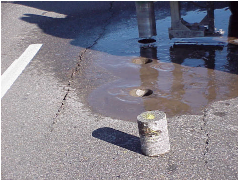
Figure 2 Coring in the Wheelpath of the Site with Distress
