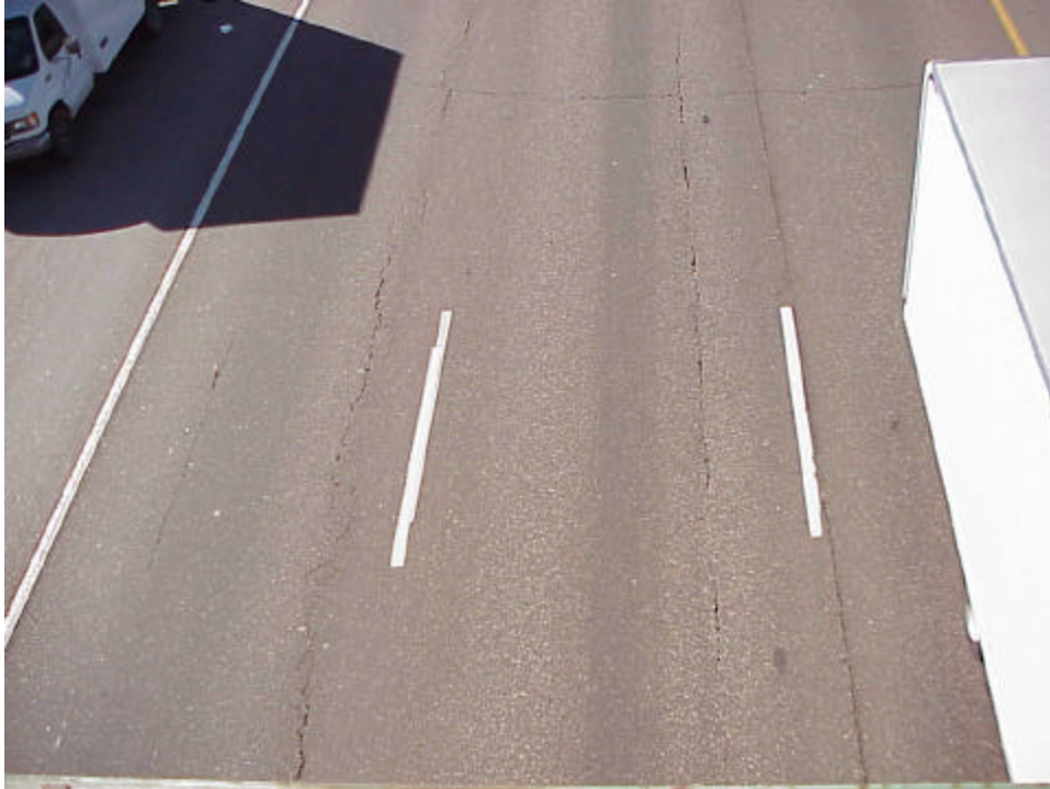
View of the outside lane and center lane just north of where the cross section slab was taken. The vehicle in the corner of the photo is carrying the saw and is parked beside the cross section site.
