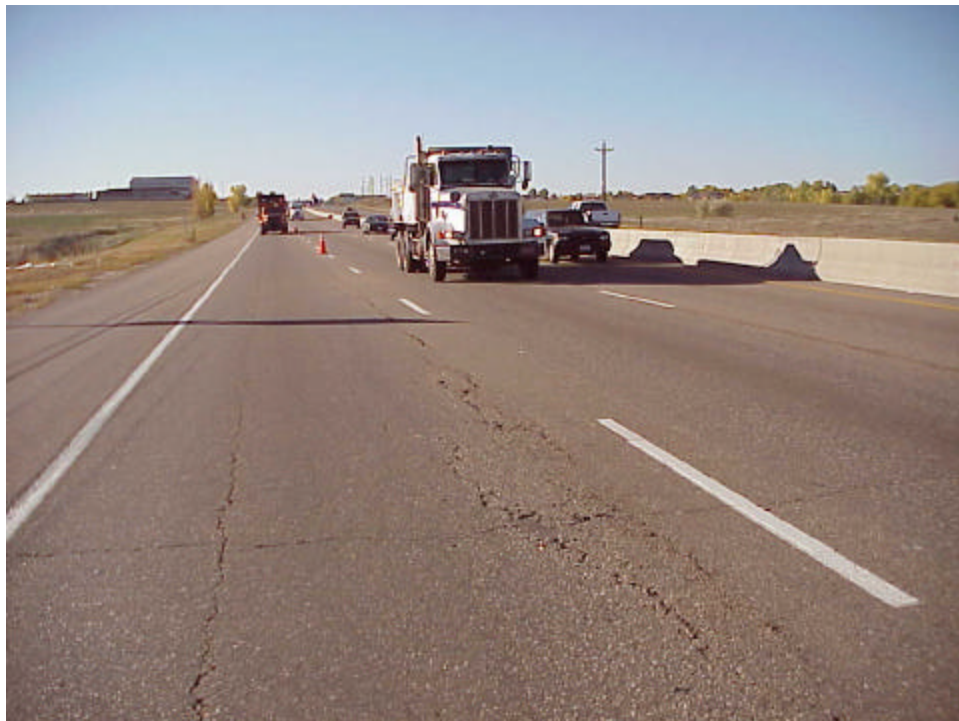
Condition of I-25 in the vicinity where the cores were taken in the distressed site.
