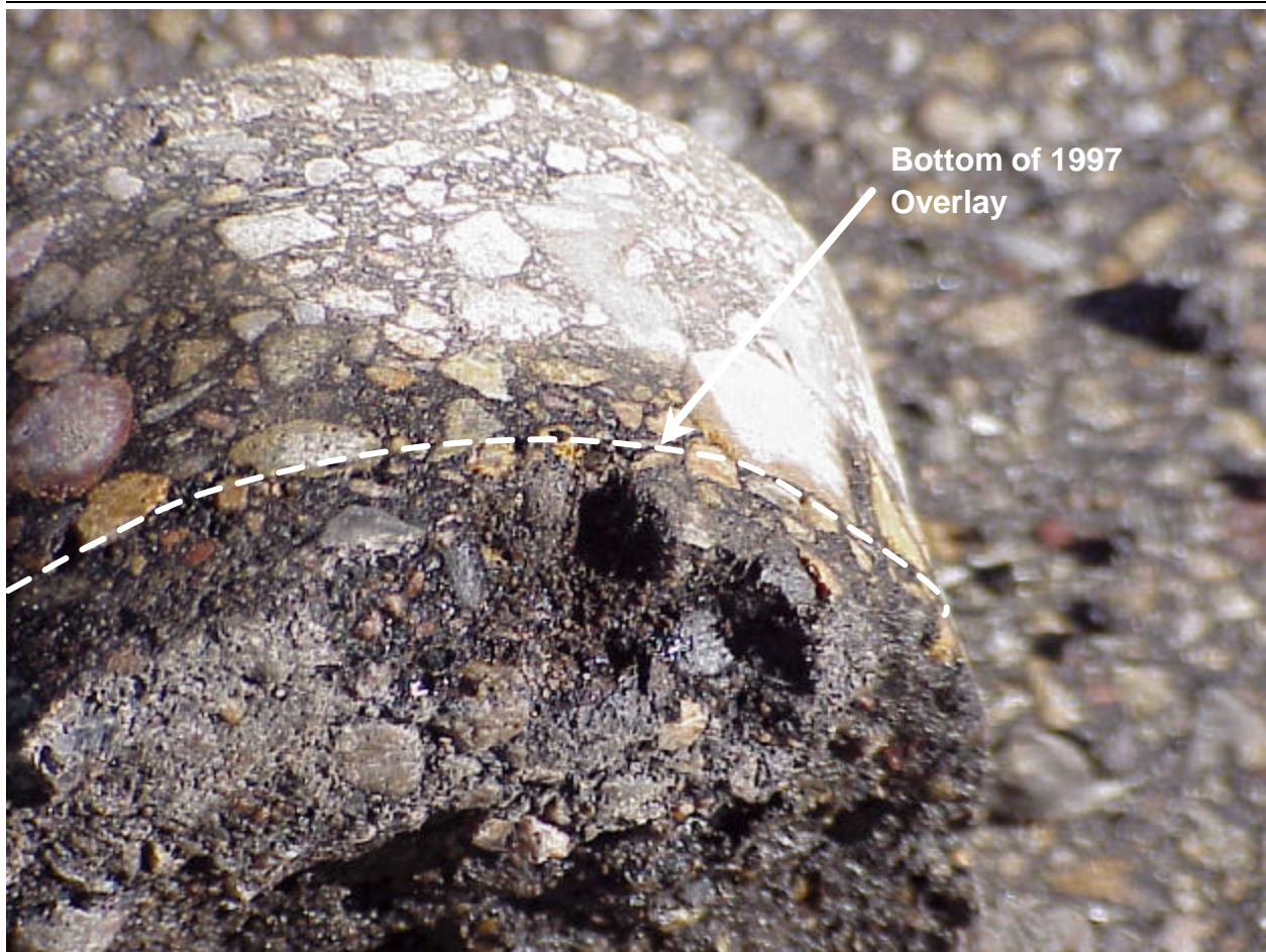
Figure 11 Bottom of Core Showing Signs of Stripping in 1984 Overlay Mixture
