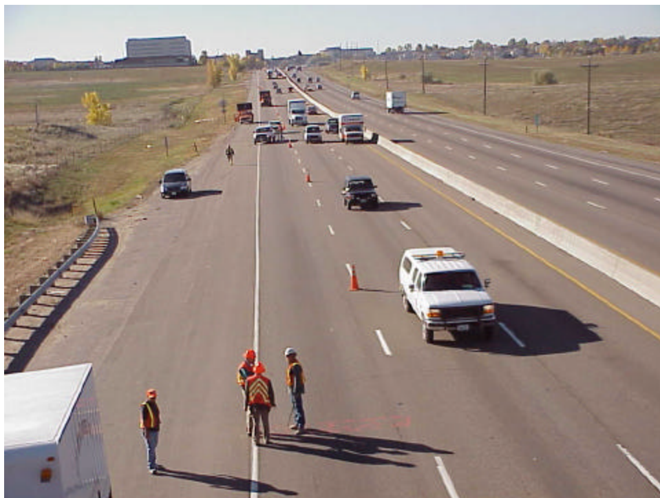
View looking south of the distressed sampling site. Location of the cross section is where the three people are standing on the lane. Coring site is about 400 feet further south where the white half ton is parked diagonally across the lane.
