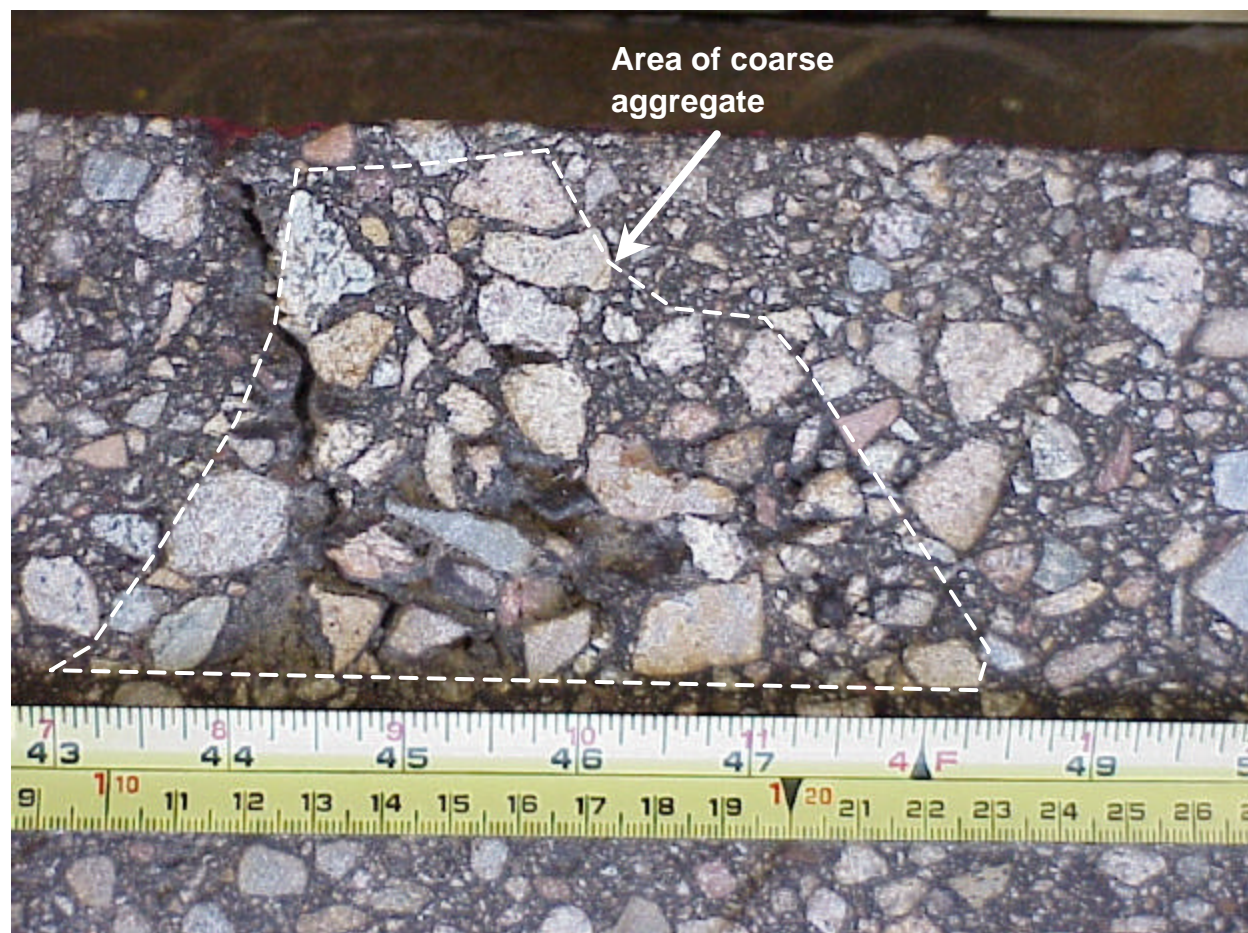
Figure 8 Close-up Cross Section at Crack Beside Right Wheelpath
