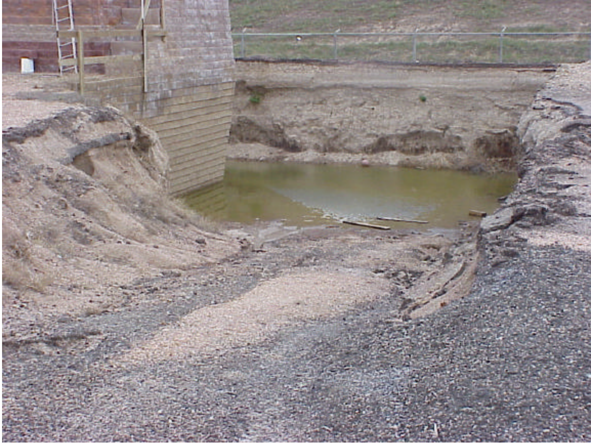
Photo 3. Lower Portion of the Abutment Structure. Note the negative batter. This was done only on the east side of the abutment and only below the ground level.
