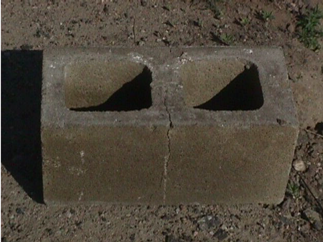
Photo 12. A Vertical Crack in a Block from the Abutment Structure.
