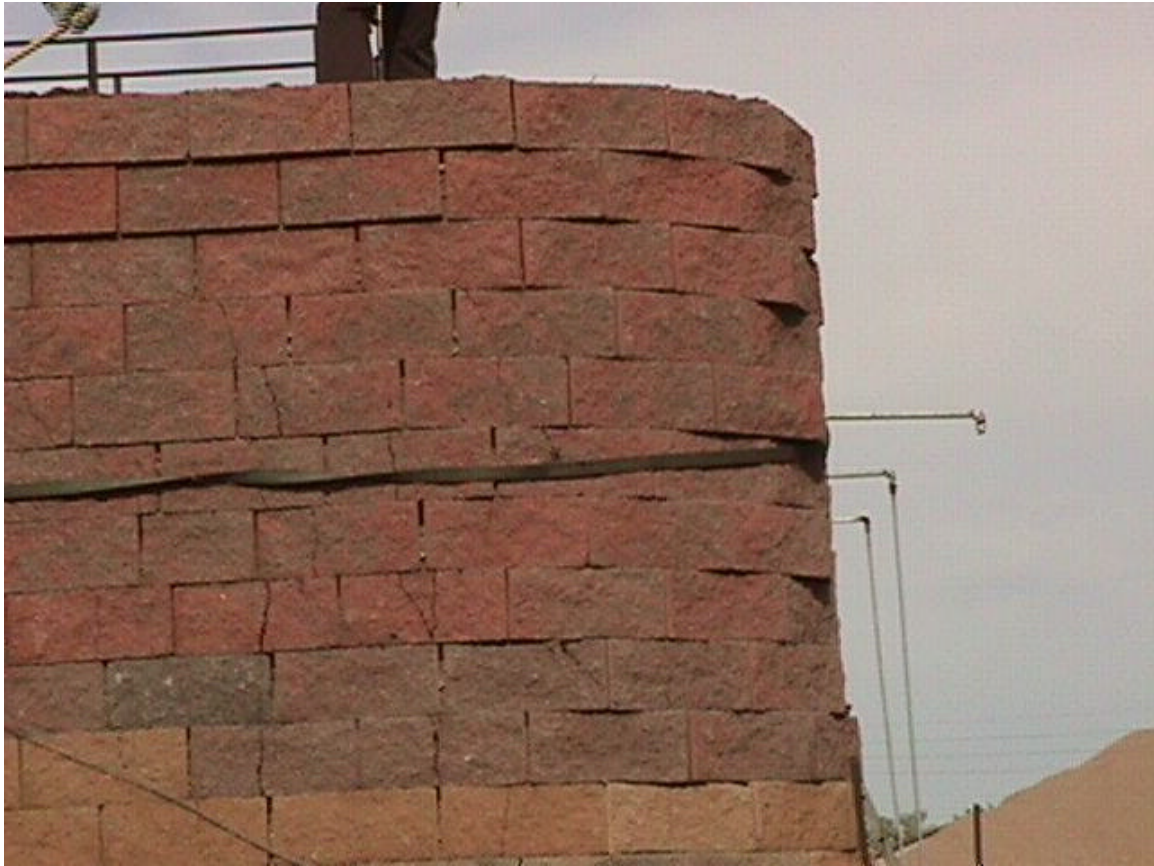
Photo 6. Excessive Movements of the Top Rows of Blocks on the Outer Pier.
