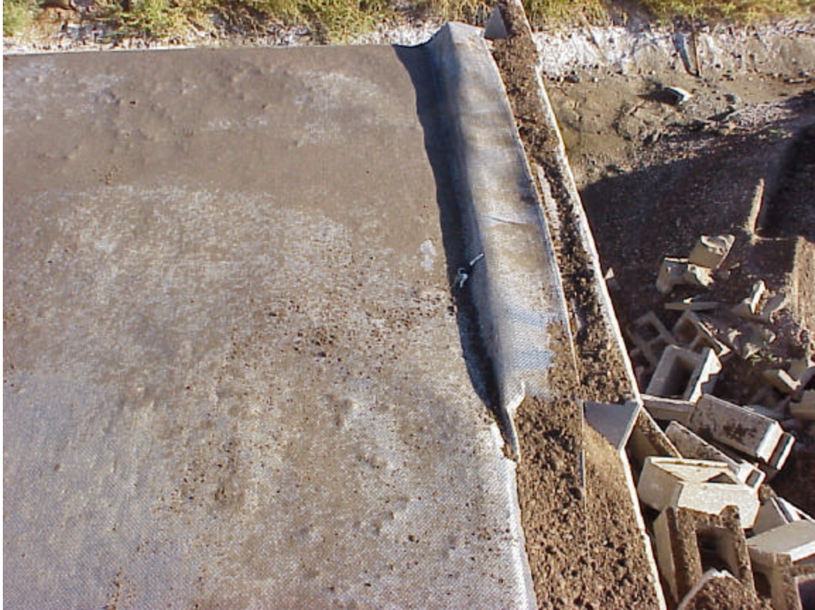
Photo 11. Geotextile Sheet During Dismantling of the Inner Pier. No damage to any of the fabric sheets was observed in any of the structures even at locations where the fill had settled considerably.
