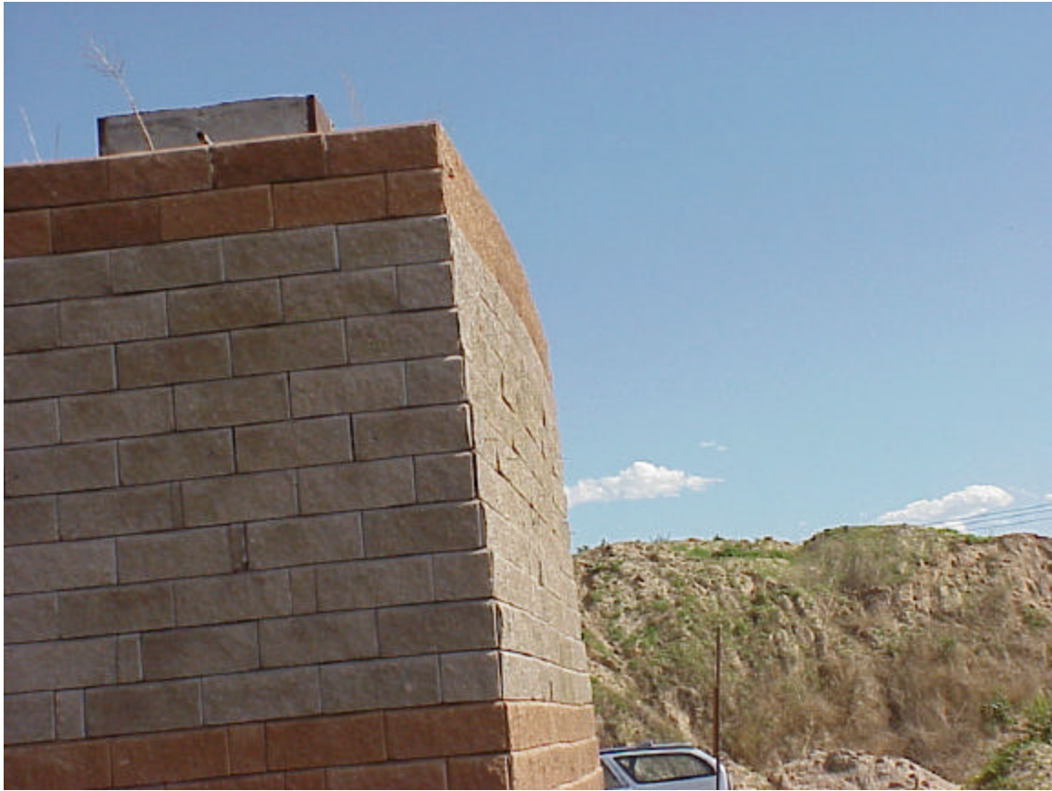
Photo 4. The Center Pier Structure. Note the outward bow of the top several rows of blocks.
