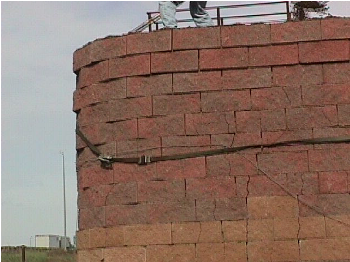
Photo 7. Excessive Cracking of the Facing of the Outer Pier Note that all cracks are vertical and they are aligned with joints in layers below or above the cracked blocks.
