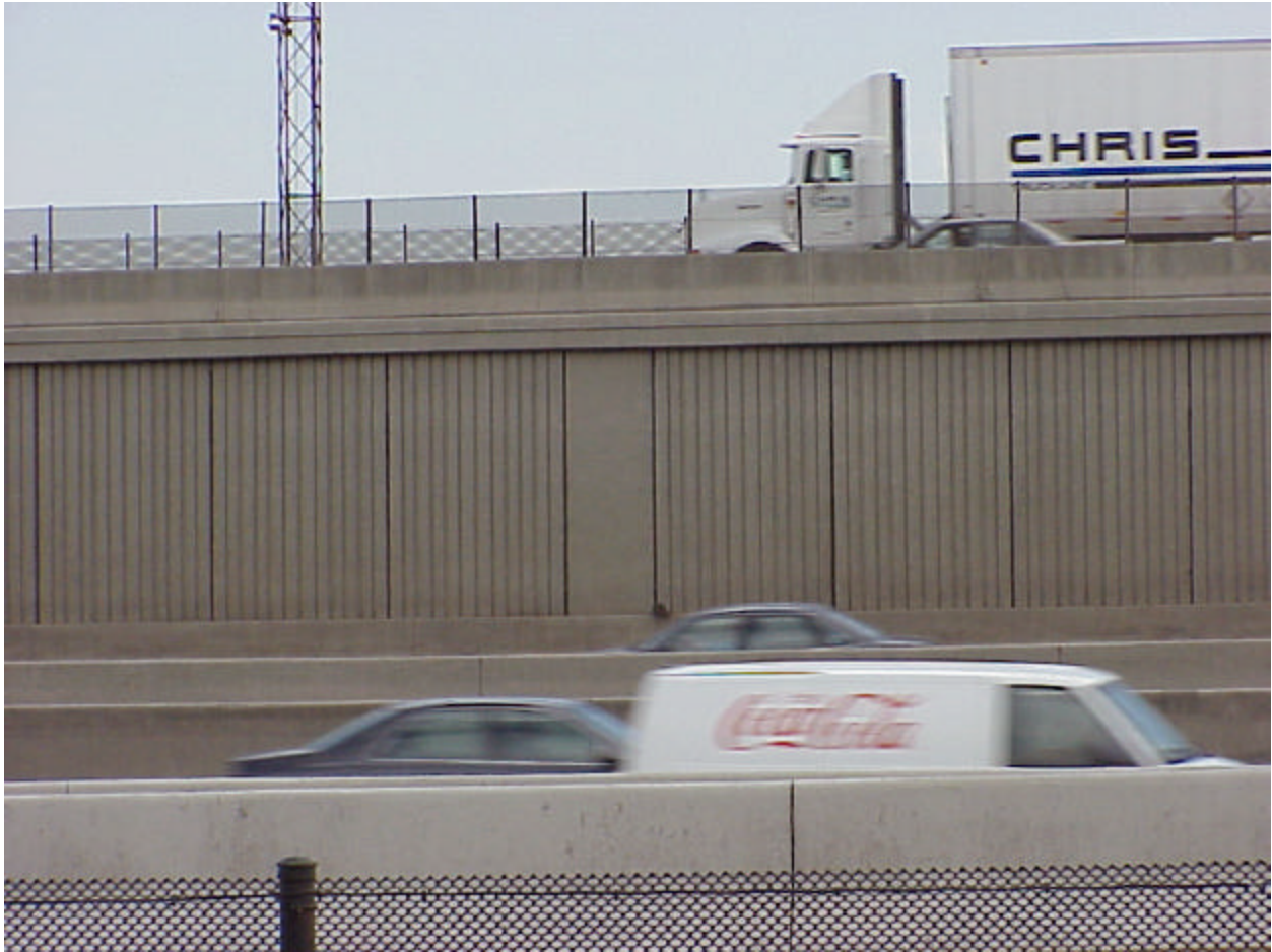
Figure 1.2. Picture of the Completed I-25/I-70 MSE Wall with Independent Full-Height Facing in Denver, Colorado.
