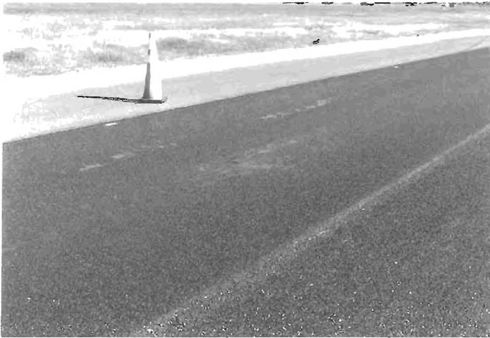
Figure 11. Limited problems with draindown were encountered.
