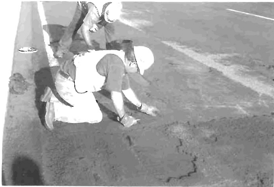
Figure 19. The exposed membrane was removed.
