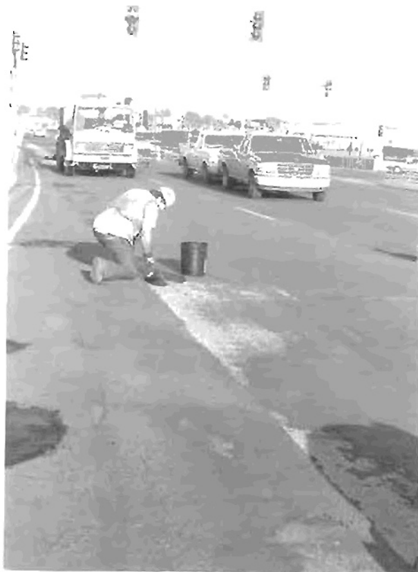
Figure 20. A cold-pour material was used to cover the area where the membrane was removed.
