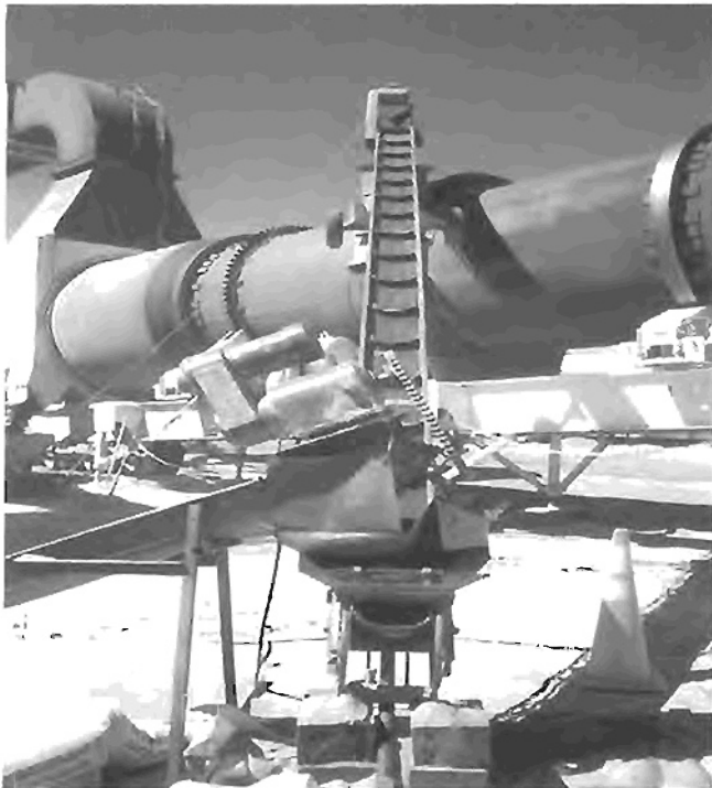
Figure 6. Conveyor system used to add Vestoplast S and fiber pellets at the RAP collar.
