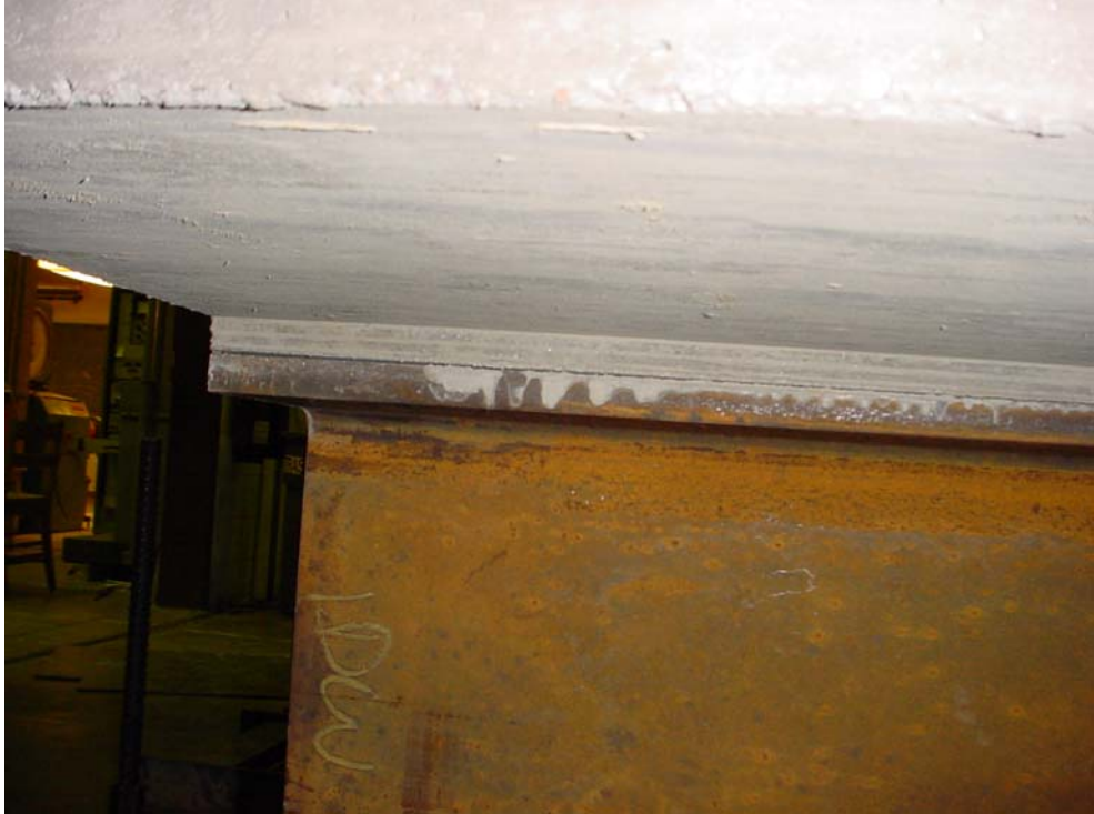
Figure 6.29 – Small Separation between the Concrete Slab and a Steel Girder
