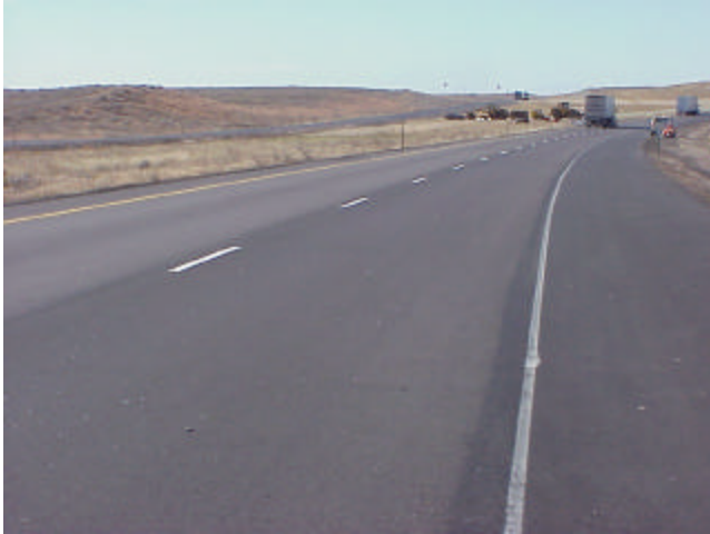
Figure 10. This photograph shows the project shortly after construction. Segregation on the surface was not apparent.
