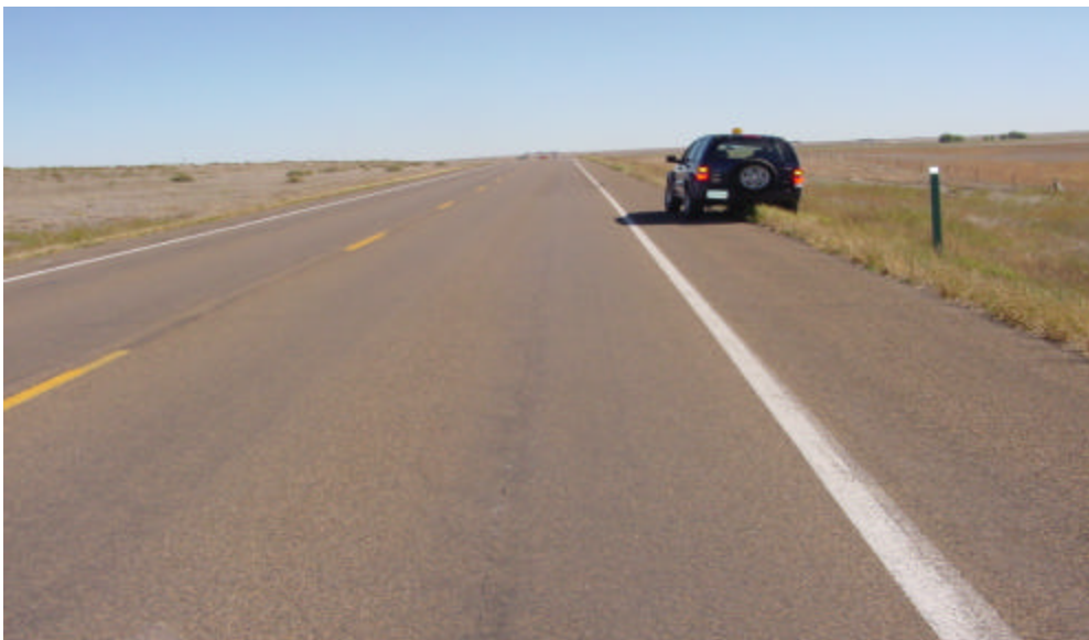
Figure 14. This distress was a reflective crack. Note the linear straightness and low severity of the crack.
