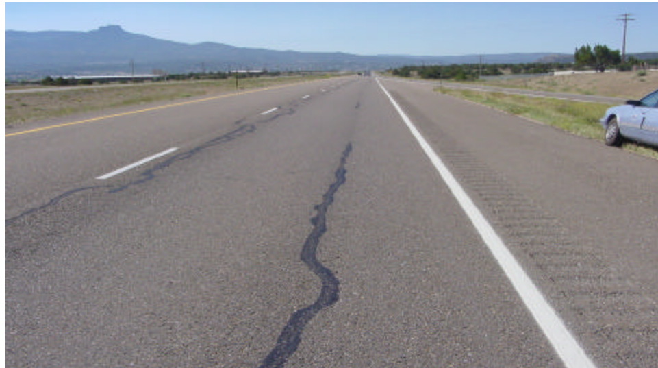
Figure 15. This crack was top-down. Although the crack is straight, the severity was enough to warrant crack sealing.
