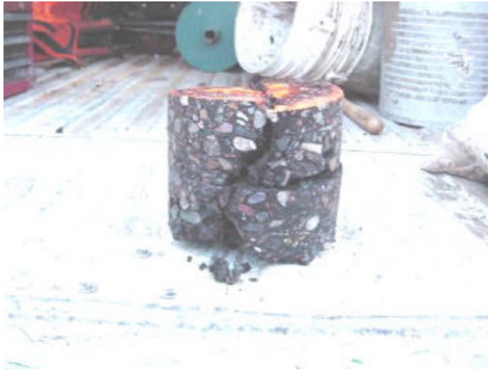
Figure 6. This crack is reflective, as it goes through the entire thickness of the pavement
