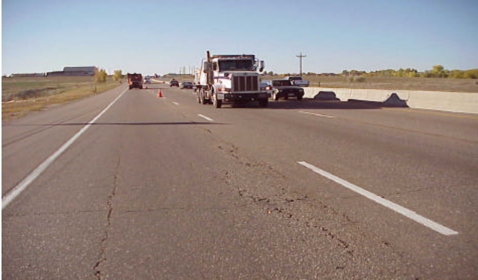
Figure 1. Longitudinal cracking was found on this project as shown in this photograph. This cracking pattern was consistent throughout the entire length of the project.
