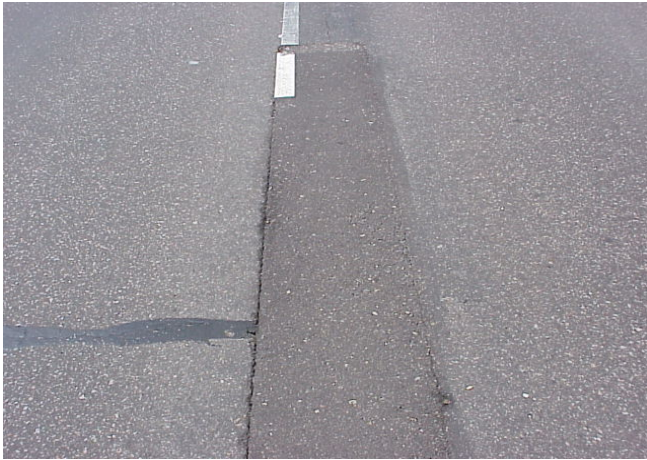
Figure 24 – This photo shows the initial longitudinal joint crack on the left. Then the contractor milled and filled one foot to the right of the crack. Eventually this pavement cracked on the edge of the 1-foot mill and fill, creating 2 cracks.
