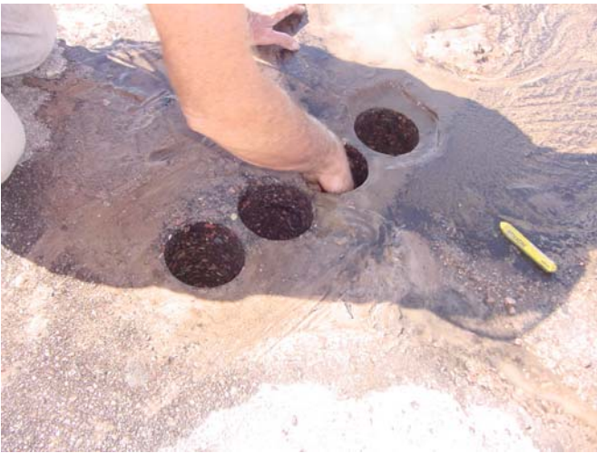
Figure 20 - In order to determine the lateral extent of stripping, additional cores were obtained at six-inch intervals transversely to the construction joint.
