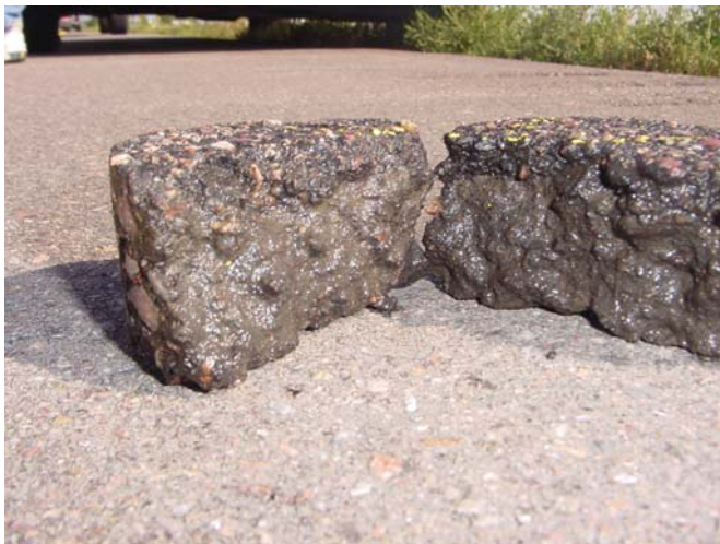
Figure 18 - Lack of AC as result of stripping at the construction joint.
