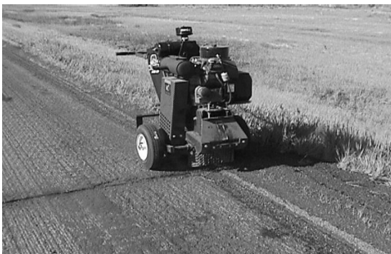
Figure 10 – Equipment used to rout the crack prior to filling it with sealant.
