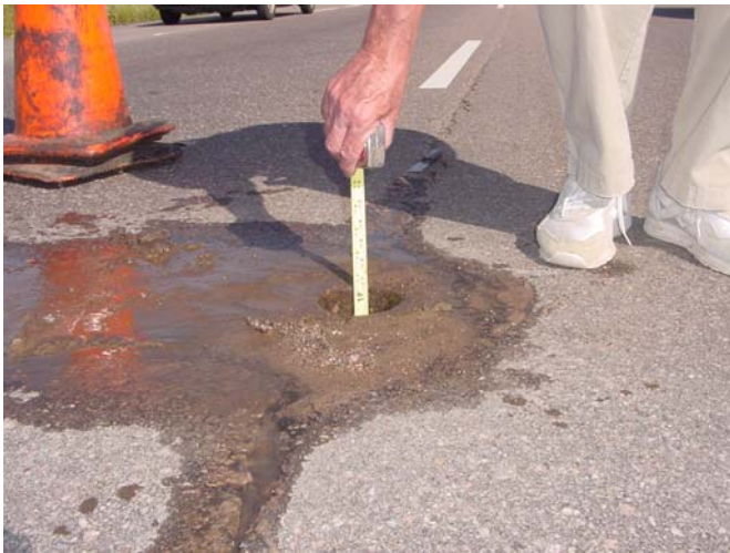
Figure 17 - Full-depth (11inch) pavement with exploratory core sample removed. Stripped aggregate material can be seen adjacent to the core hole.
