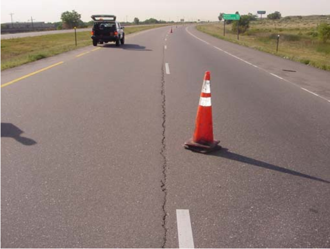
Figure 14 – Longitudinal construction joint failure at end of warranty period. Longitudinal crack is evident throughout most of the project.
