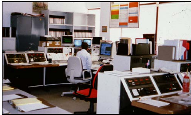
Figure A-9 New Dispatcher's Console
