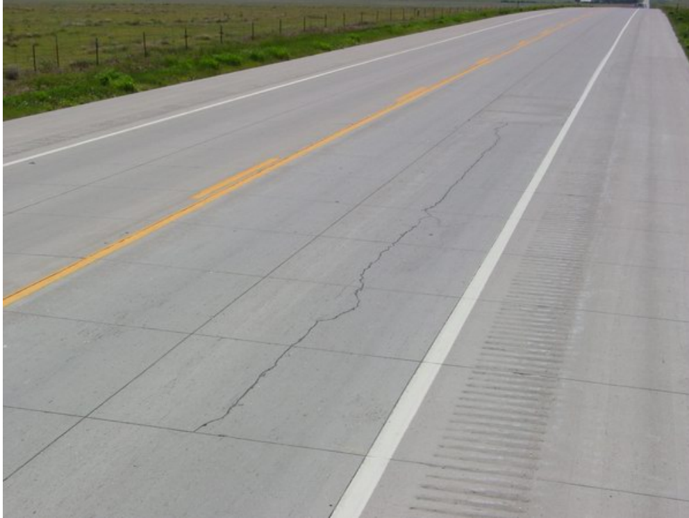
Figure 4.9. Typical Cracked Slab Conditions Observed at the U.S. 287 Lamar Site
