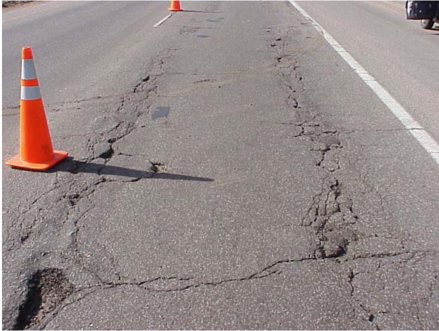
Figure B.1. Fatigue Cracking Observed in Test Sections 1 and 2
