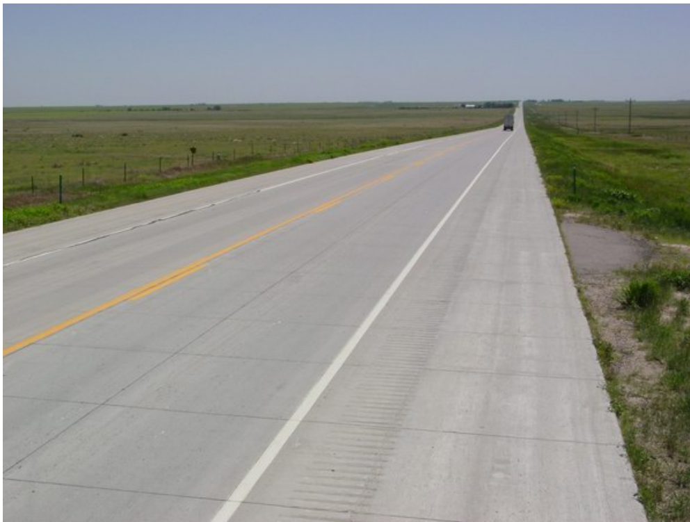
Figure 4.8. Typical Pavement Conditions Observed at the U.S. 287 Lamar Site
