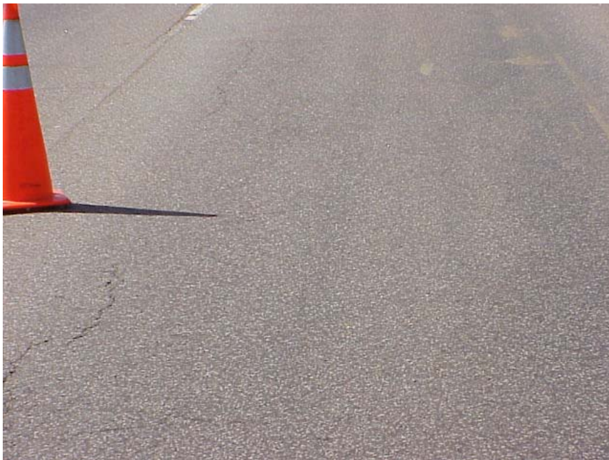
Figure B.2. Typical Conditions Observed in Test Sections 3 and 4
