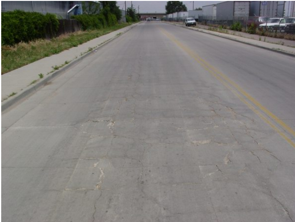
Figure 4.5. Stop Sign Approach Distressed Area Observed at the U.S. 85 Site
