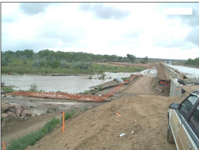
Figure 1.6. View of failed Pinon Bridge detour on Fountain Creek. Spring 2004 (CDOT Region 2).
