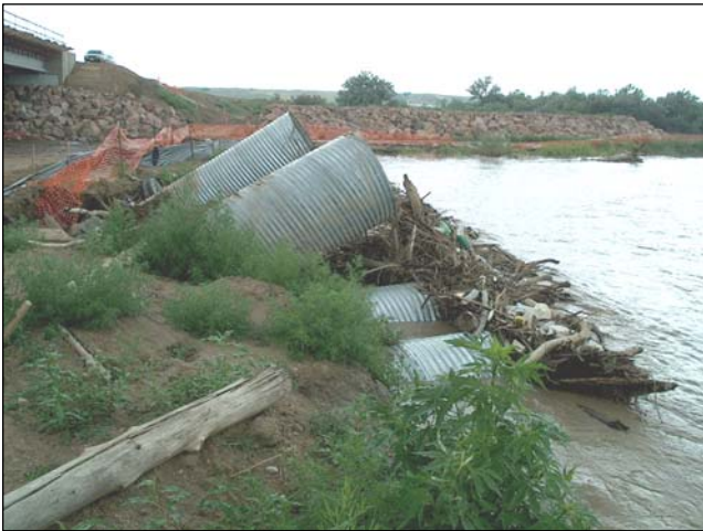
Figure 1.5. View of failed Pinon Bridge detour culverts on Fountain Creek. Spring 2004 (CDOT Region 2).
