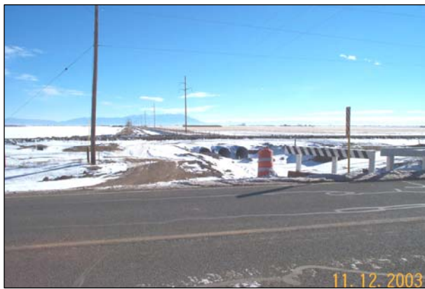
Figure 1.2. Construction of detour drainage structure. Three 60-inch pipes under Prairie Bridge detour (CDOT Region 5).
