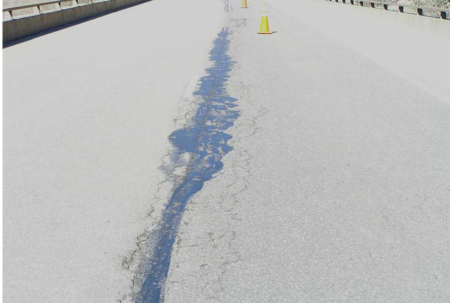
Figure 14. Alligator Cracking Developed Along Both Sides of the Construction Joint in Test Section 2.
