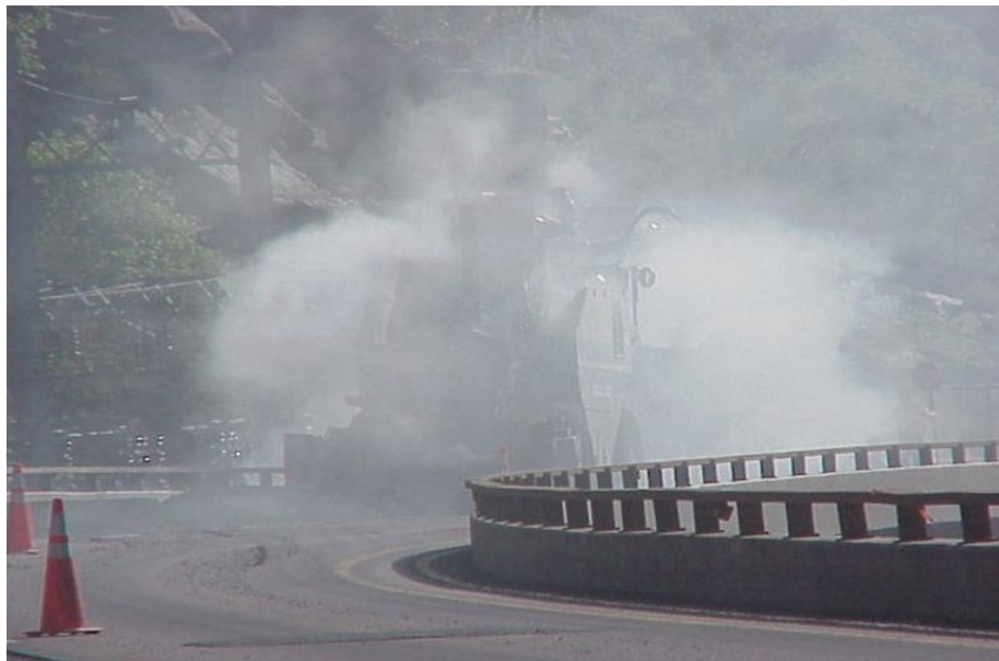
Figure 5. There Is a paver Hidden in the Smoke Behind the Transfer Vehicle. High Mix Temperatures Were Required.
