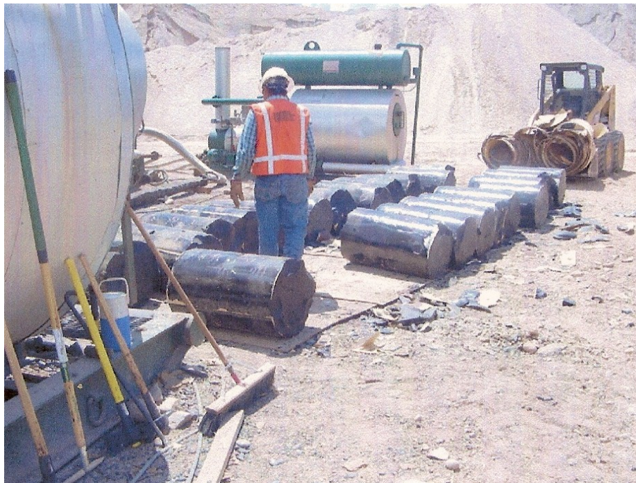
Figure 7. Trinidad Lake Asphalt Ready to Blend in Asphalt Tank
