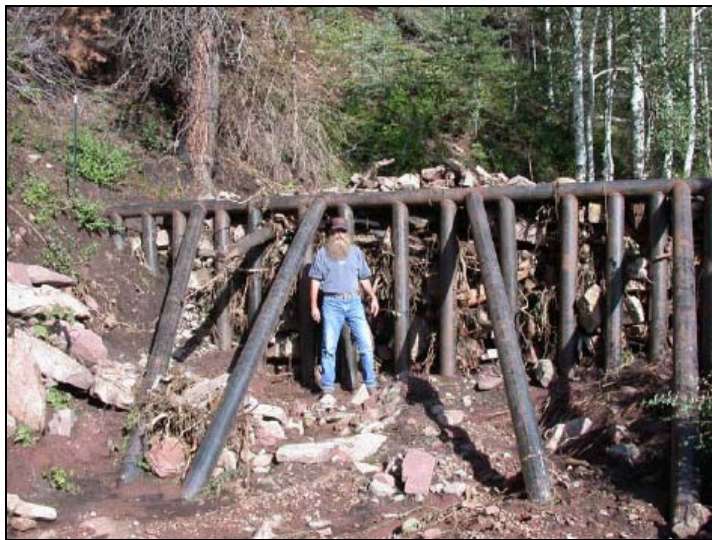
Figure 4 – A debris rack above Lemon Dam (near Durango, CO) successfully contained coarse material from a debris flow after the Missionary Ridge Fire of 2002 (from Florida Water Conservation District, 2003).
