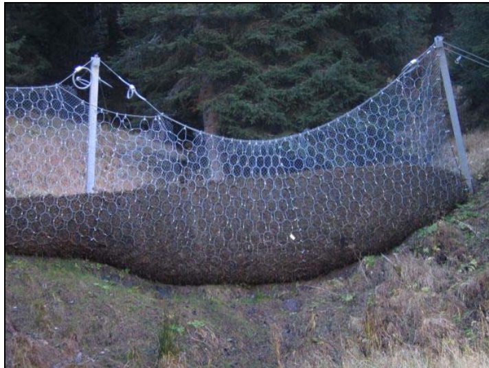
Figure 3 – The use of a high tensile-strength ring net to contain a debris flow (from www.wsl.ch )
