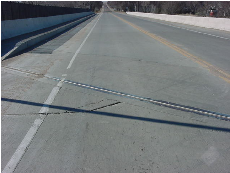
Figure C.14. Photos of Structure G-22-BX in Region 1.
