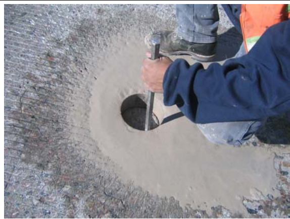
Figure 13 - Coring Concrete Samples on Bridge G-22-BJ. The Core Was Broken in the Traffic Lane
