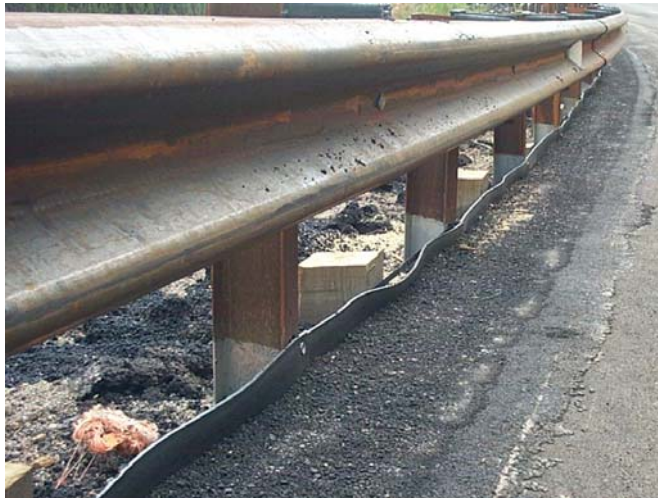
Figure 6. The edge of the pavement was placed and compacted by hand.
