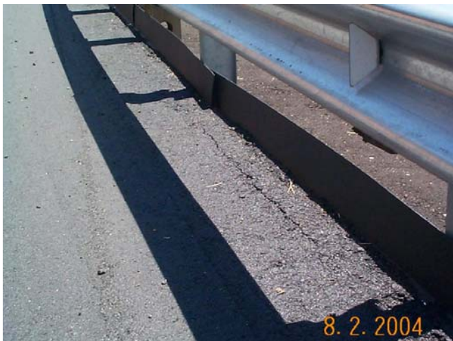
Figure 14. Cracks along the edge of the HDPE on US-24.
