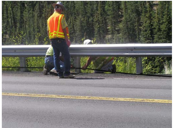
Figure 13. Steel band was installed to provide support for the DFC between posts.
