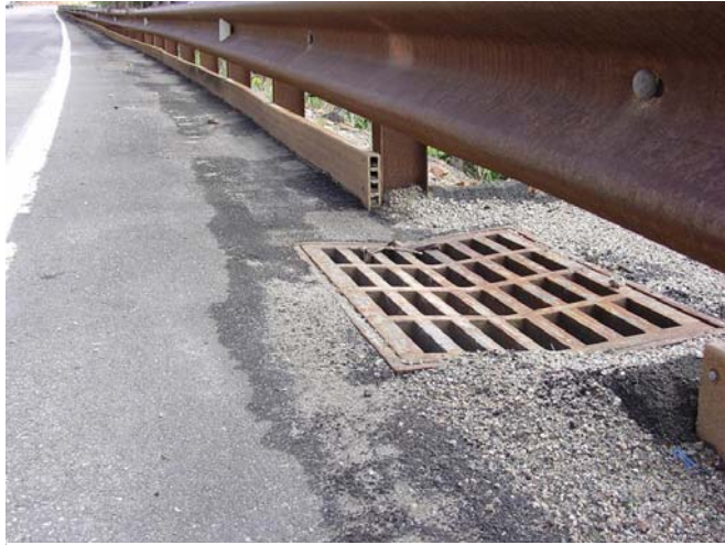
Figure 19. A hollow section of composite lumber curb ends at a drain.
