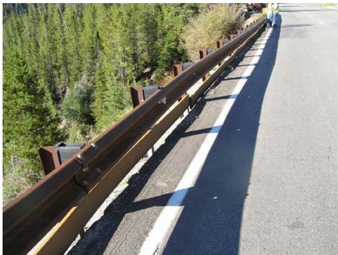
Figure 7. Slight movement of the guardrail can render the curb completely ineffective.
