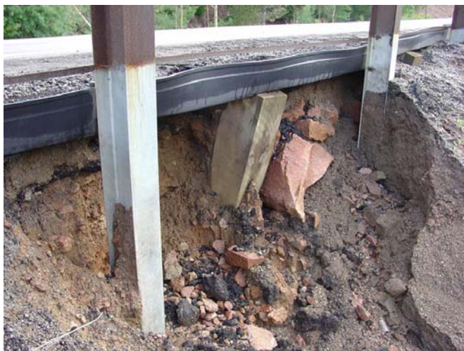
Figure 9. Without the support of the DFC, the edge of the pavement would have collapsed.
