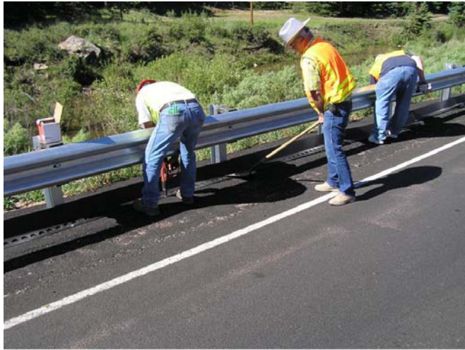
Figure 10. Holding DFC tight against the post base and the pavement with a shovel.
