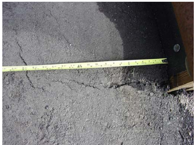
Figure 15. Cracks are developing at the end and along the edge of the DFC on US-50.
