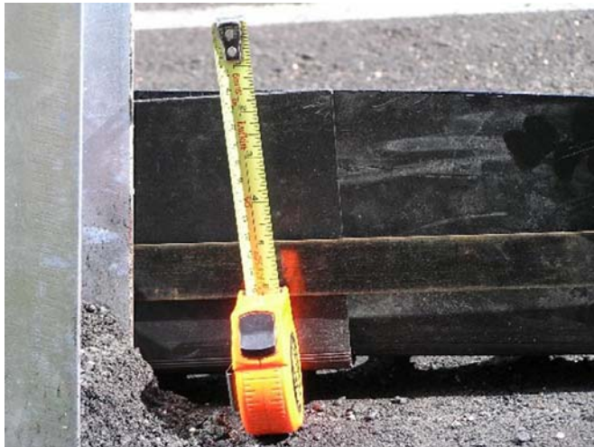
Figure 11. Air gaps between the curb material and the pavement surface.
