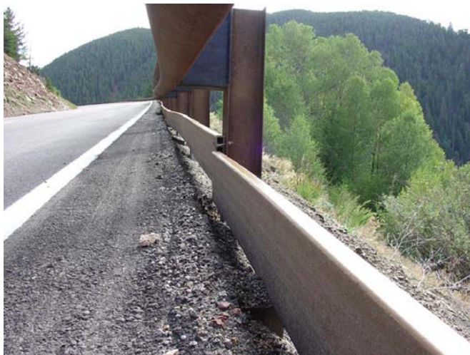
Figure 20. A small movement of the guardrail separated this curb from the pavement.
