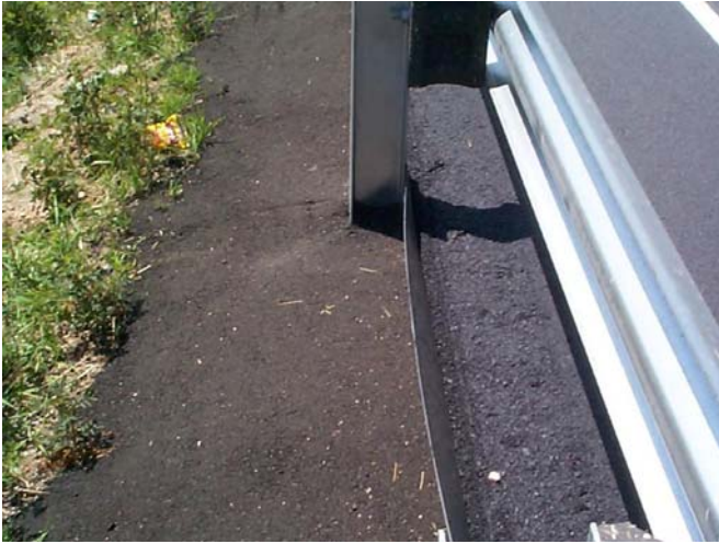
Figure 12. Wavy curb face between guardrail posts is mainly a cosmetic problem.
