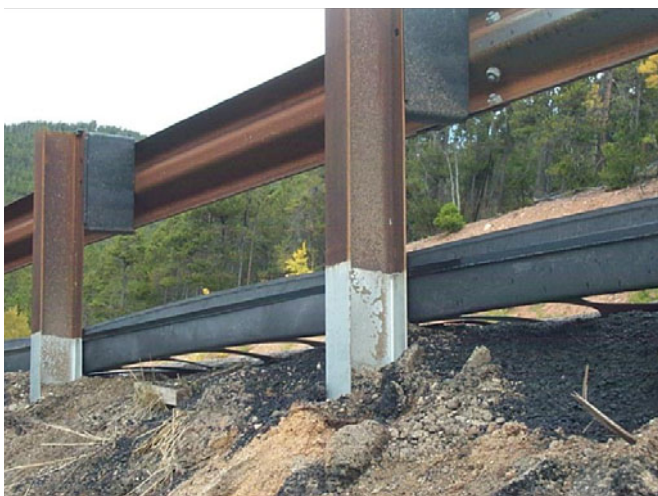
Figure 24. Inadequate base for the DFC.
