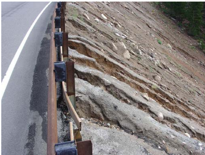
Figure 5. Severe erosion can occur very rapidly.
