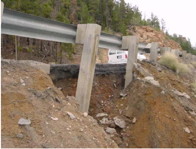
Figure 1. Dangerous erosion on US-50.
