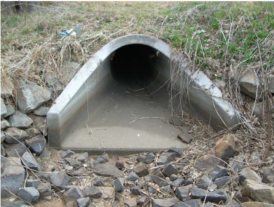
Culvert 4. East Boulder Ditch. This is a round concrete culvert and the smallest diameter (1 m) of all the culverts.
