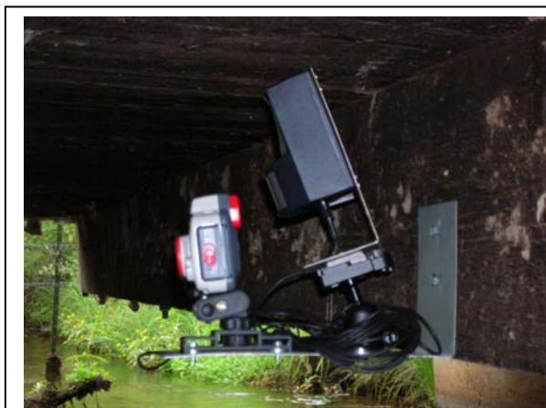
Camera (left) and monitor (right) installation. They are placed on a metal platform attached to the culvert wall.
