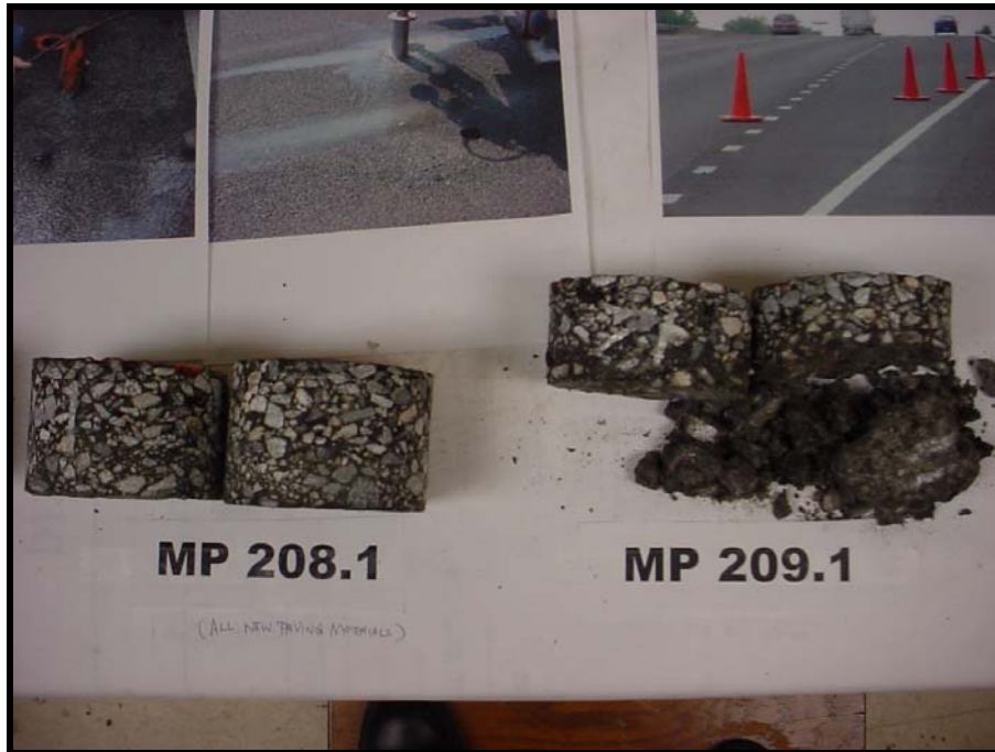
Core samples showing stripping from moisture damage
