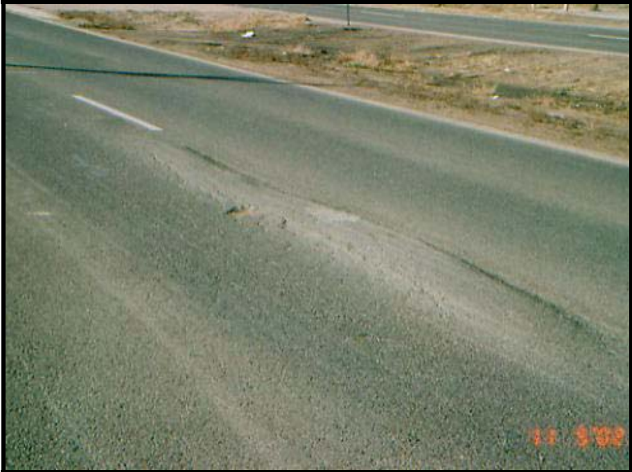
Rutting and shoving evident during the remediation construction
