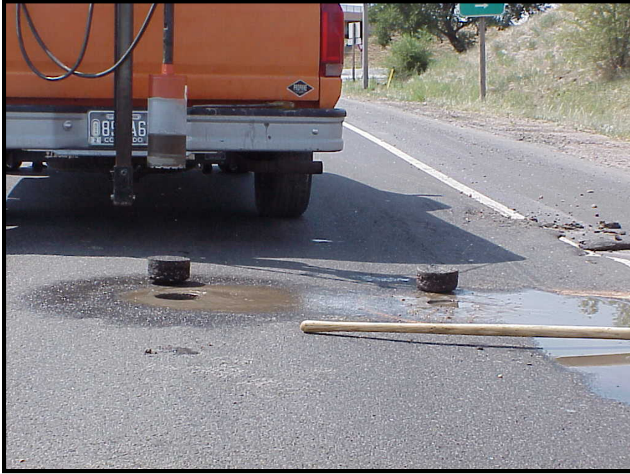
One to two inch ruts in the number 2 lane where truck traffic was concentrated
