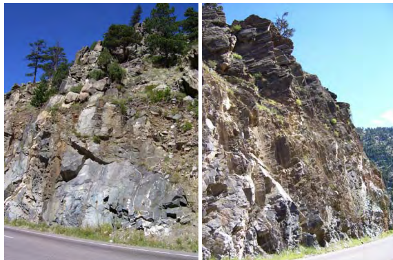
Figure 2.35: Example of mitigation effectiveness graded as D: Picture was taken on CO 14 in Larimer County. Mitigation consisted of mesh. The mesh is confined to only one section of the slope. Large blocks can easily dislodge and would likely tear the mesh from the slope.
