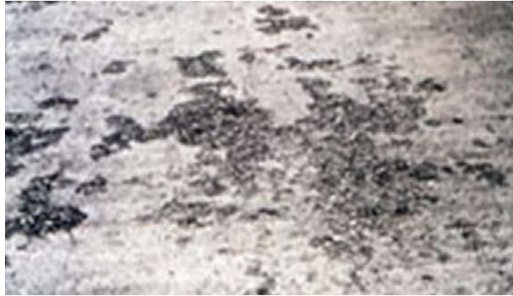
Figure 3. Concrete surface scaling (PCA, 2008)
