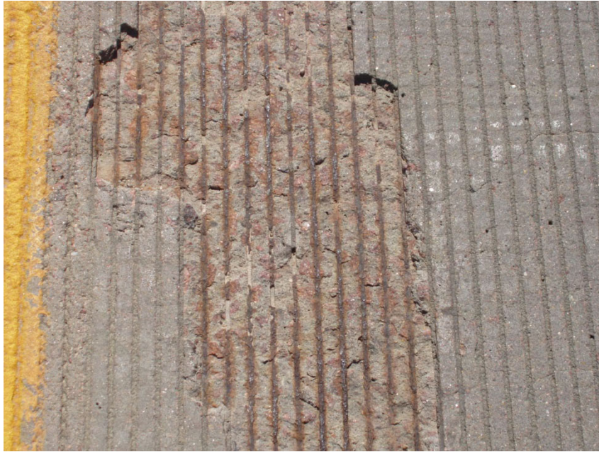
Figure 13. View of a scaling area on structure G-22-BY
