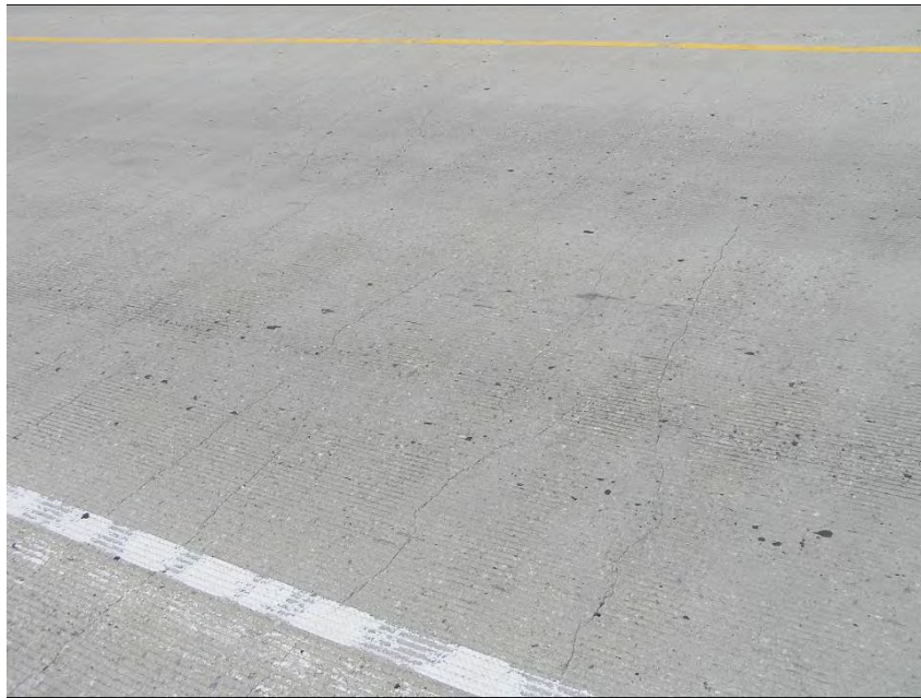
Figure 12. View of transverse cracking at structure F-15-BZ
