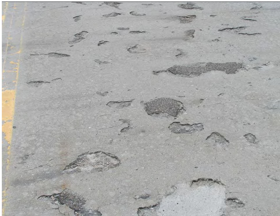
Figure 9. View of scaling on structure D-14-I
