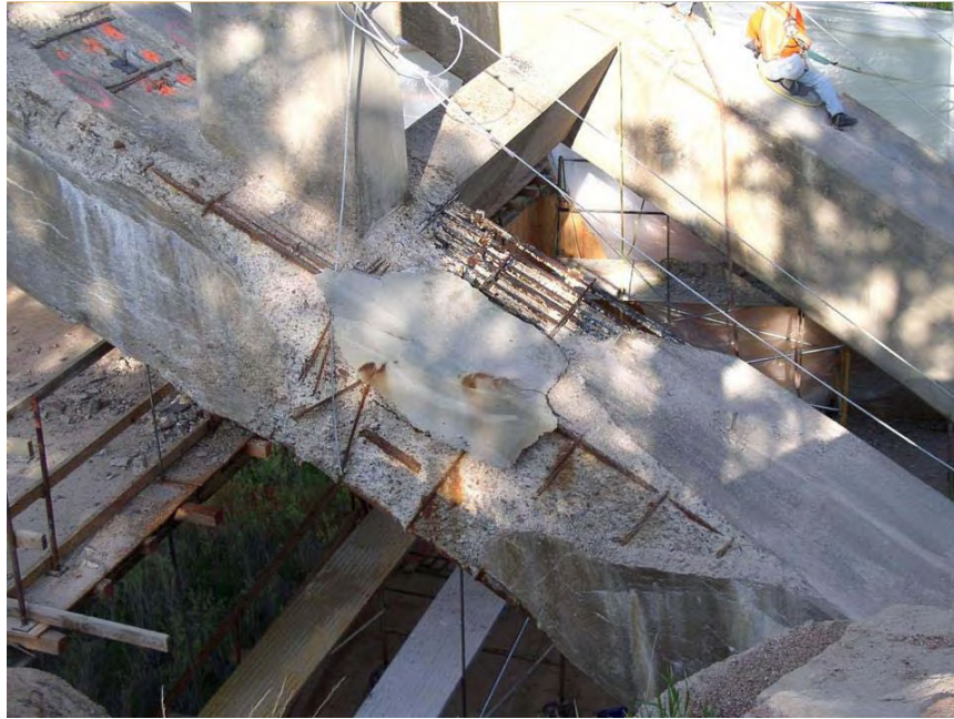
Figure 1. Freeze-thaw deterioration at Castlewood Canyon (Ardani, 2004)
