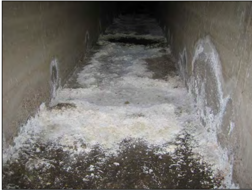
Figure 12. Concrete pipe corrosion at Site 4 (North of Walsenburg)
