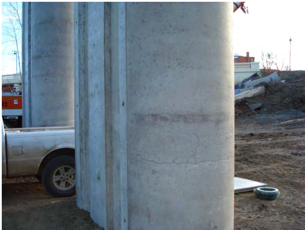
Figure 22: Pier Column Surface Defect
