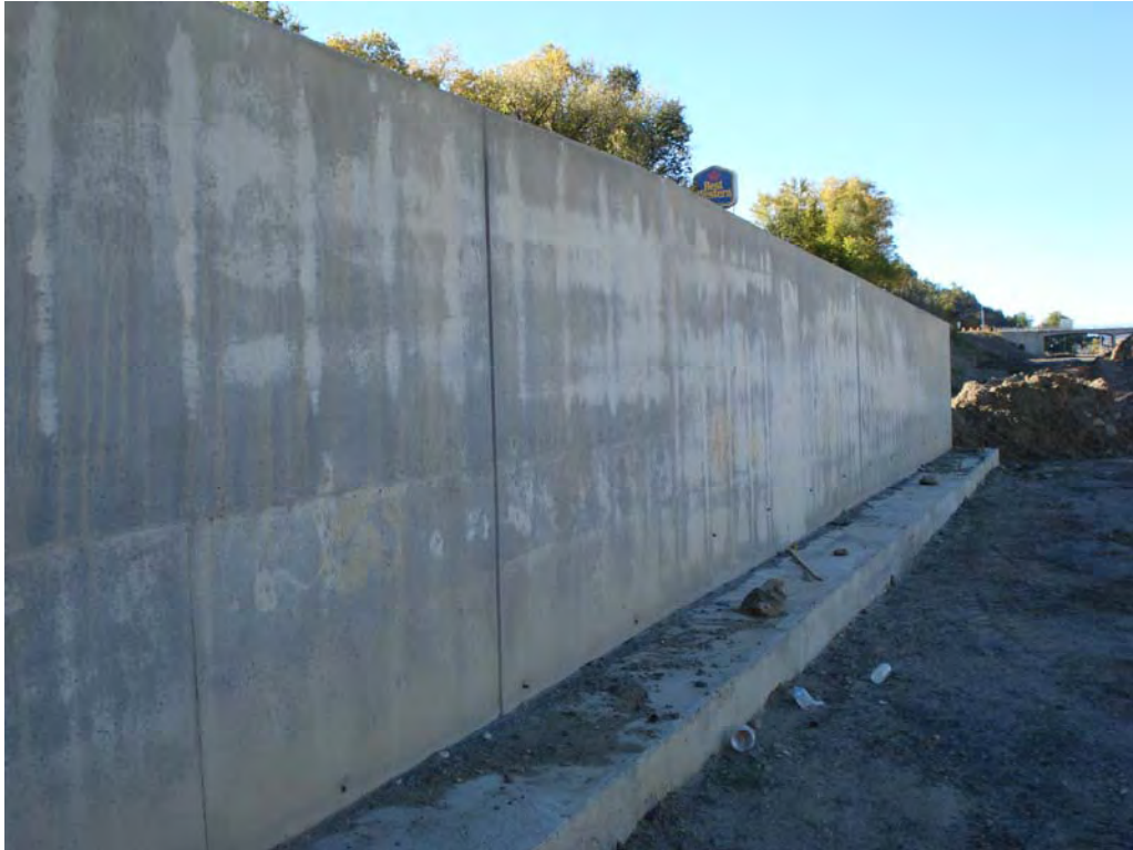
Figure 11: Discolorations on Retaining Wall
