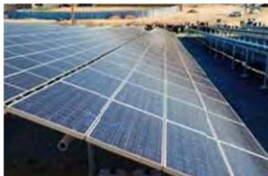
Figure 31-g. Portion of CSU-Pueblo Solar Array
