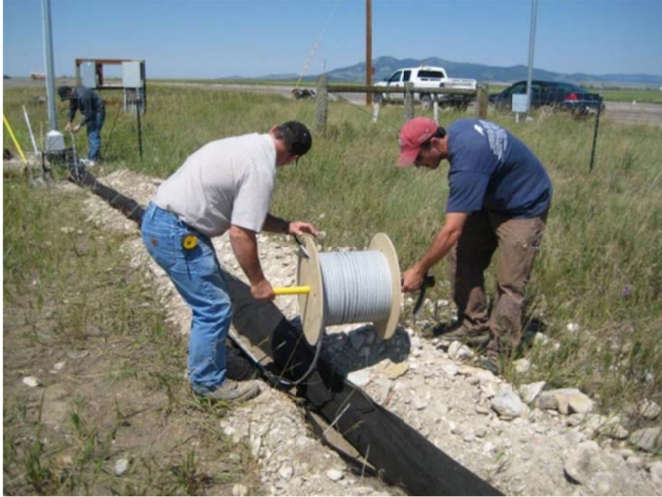
Figure 4.5: The installation of the Senstar Perimitrax® cable. The cable is embedded with sand and wrapped in geotextile (Photo: Marcel Huijser, WTI/MSU).
