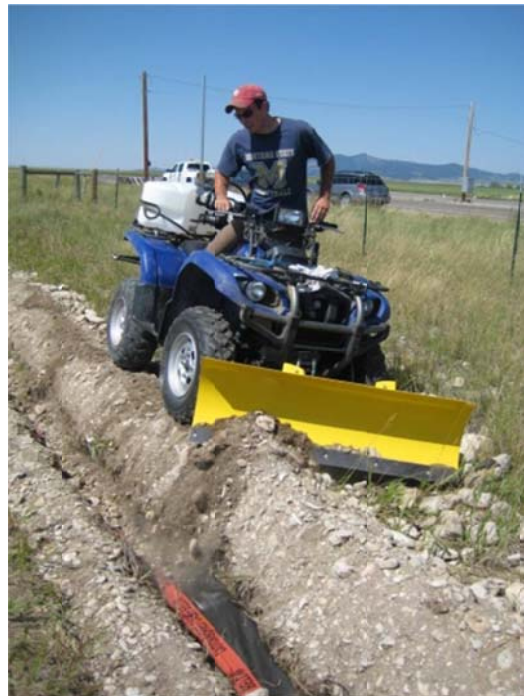
Figure 4.6: The installation of the Senstar Perimitrax® cable. Filling up the trench (Photo: Marcel Huijser, WTI/MSU).
