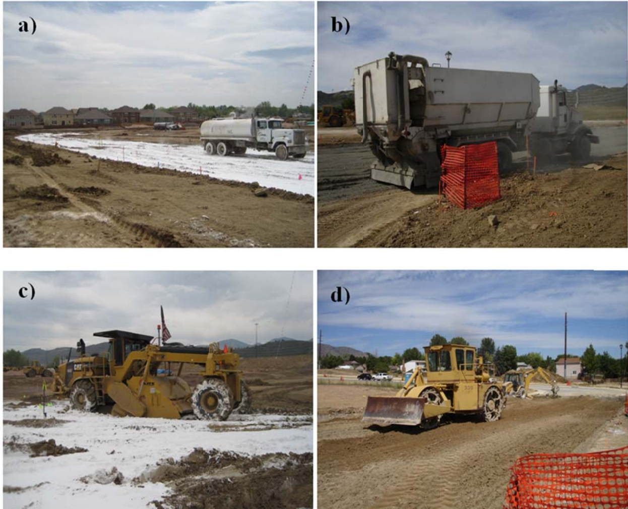
Figure 3.5: (a) Application of quicklime slurry, (b) application of cement, (c) soil/stabilizer mixing, and (d) final compaction.
