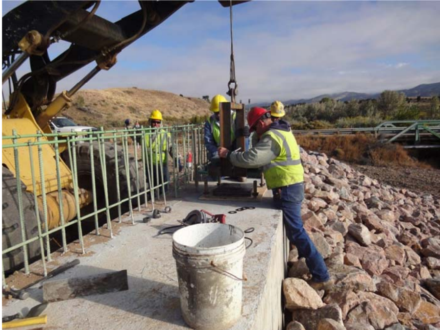
Figure 15 – Setting of Bearings (Note: A special clamping bar was used to lift the bearings.)
