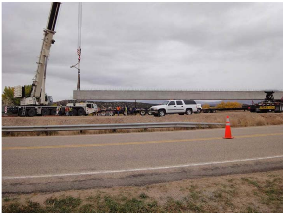
Girders for the replacement structure, N-17-Q arrived at the site on trucks. The span was too wide for a single crane to set the girders so a pair of cranes, one at each end of the structure, positioned the girders. The east end of a girder was lifted from its truck by the crane at the west abutment.
