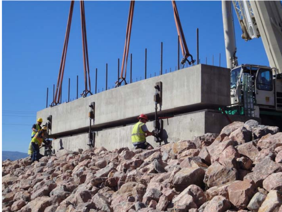
Figure 16 – Setting of cap beam (Note: The crane supported some of the cap's weight while the stays were connected and hand tightened.)
