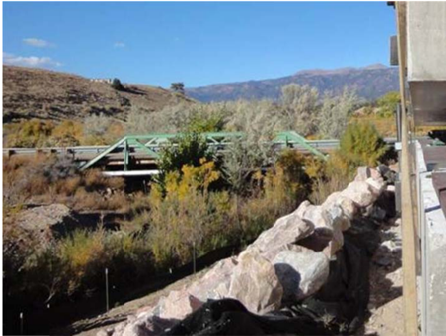
Structure N-16-L at mm 18.9 on SH-69 northwest of Walsenburg was built in 1923.
