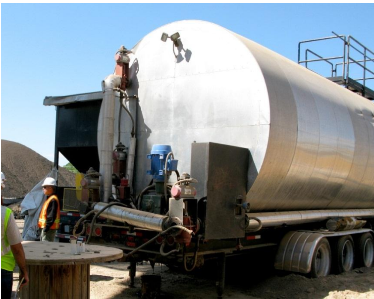
Figure 7 – EcoPath Mixing Tank
