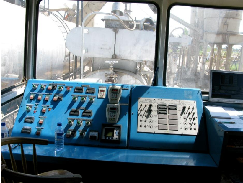
Figure 6 – EcoPath Control Room
