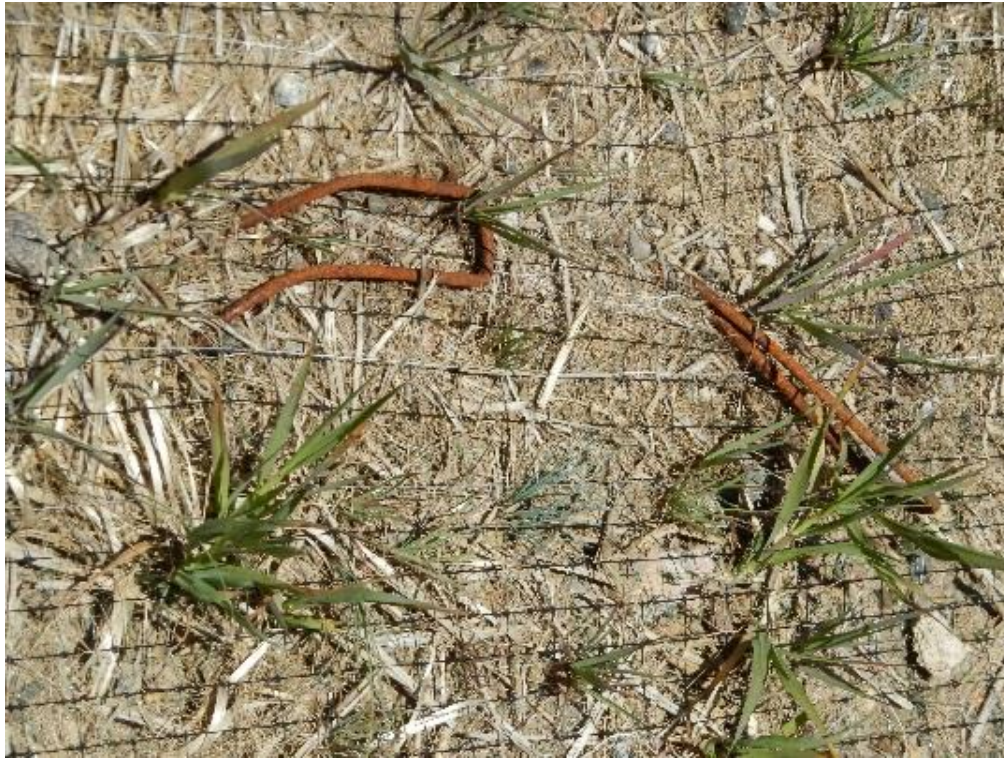
Figure 9. Blanket staples not installed completely - likely due to high soil compaction.
