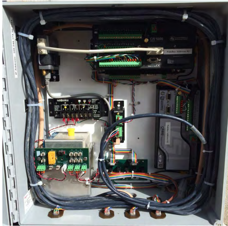
Photograph B-1. Abutment 4 vibrating wire data logger internal components.
