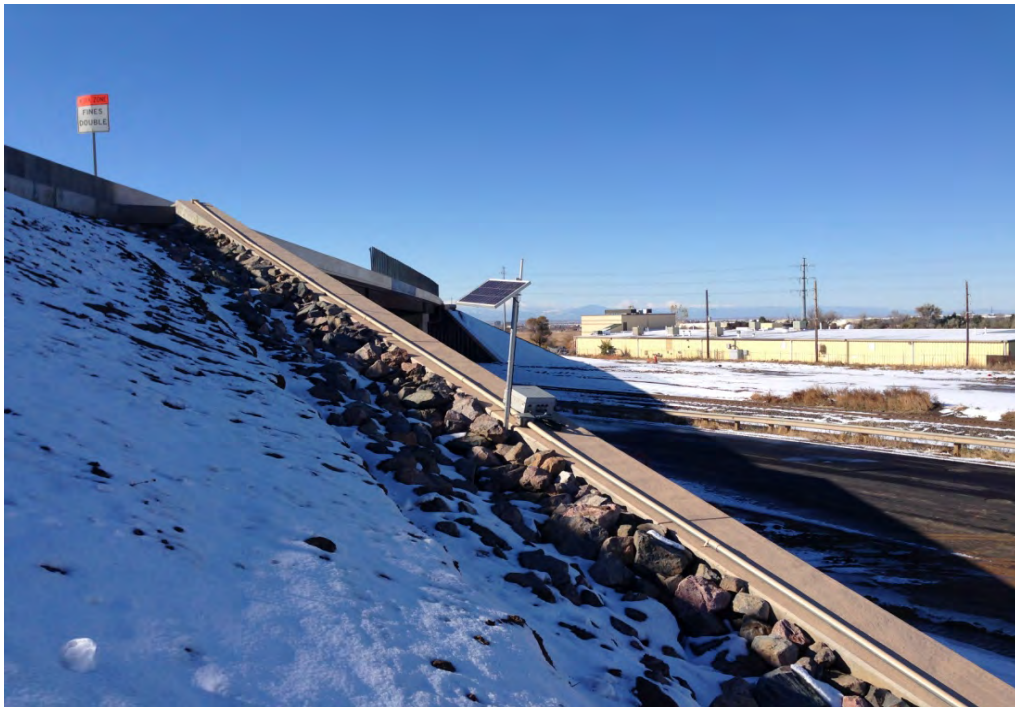
Photograph B-2. Abutment 4 vibrating wire data logger and solar panel.
