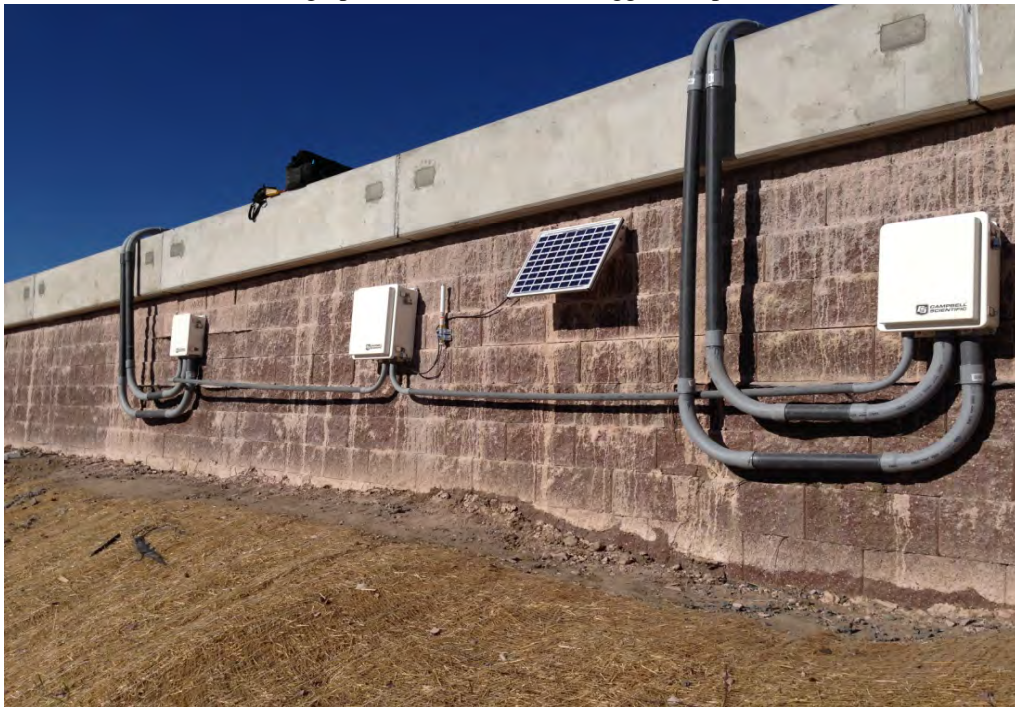
Photograph B-8. Wall DH data logger, multiplexers, and solar panel.
