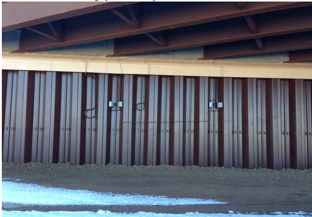
Photograph B-4. Multiplexers 1 through 4 installed on sheet pile at abutment 4.
