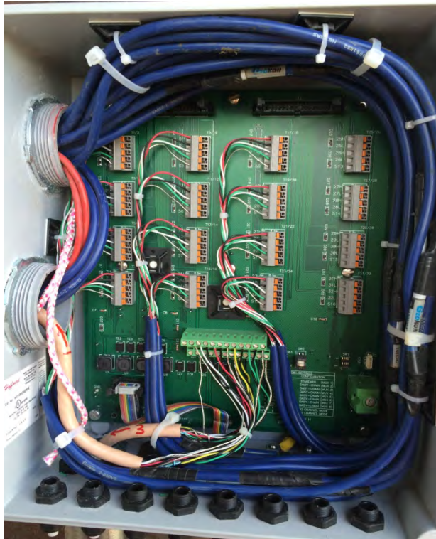
Photograph B-3. Multiplexer 1 at abutment 4.
