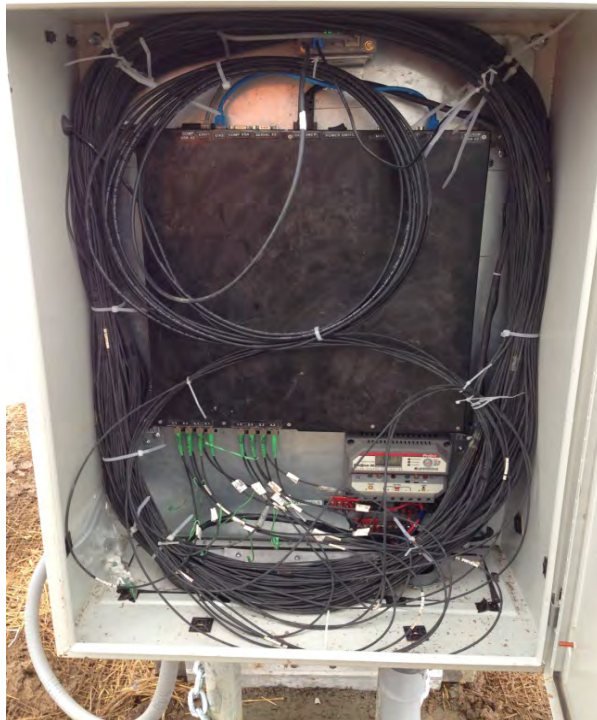
Photograph B-5. Abutment 4 fiber optic data logger components.
