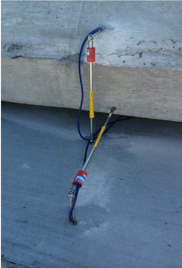
Photograph A-5. Horizontal and vertical crackmeters.
