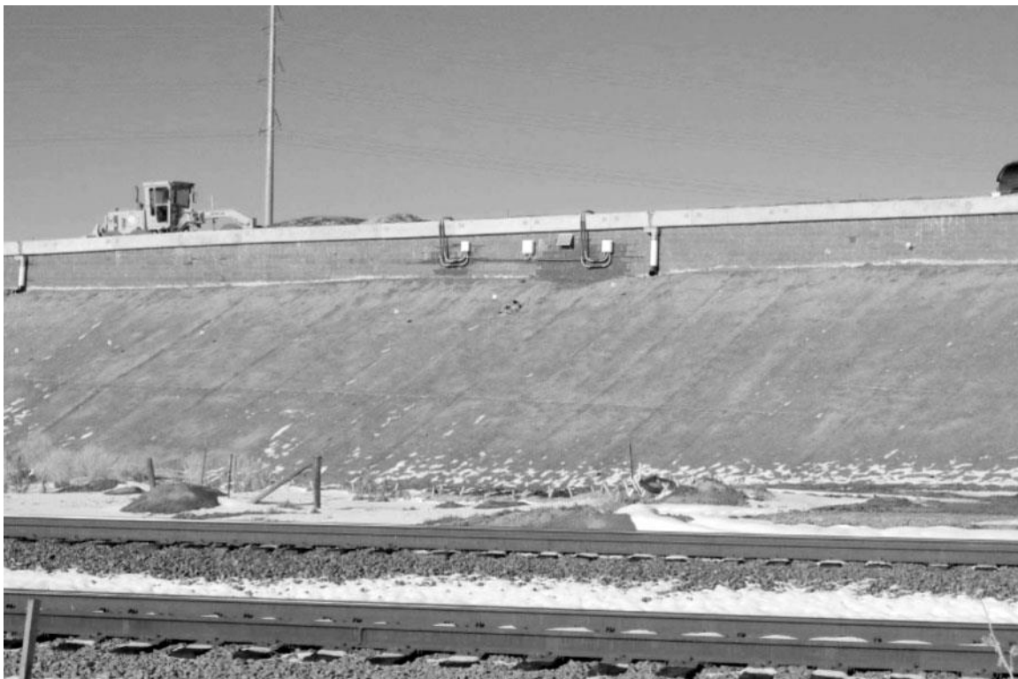
Figure 28. Photo of instrumented GRS Wall on I-70 over Smith Road
