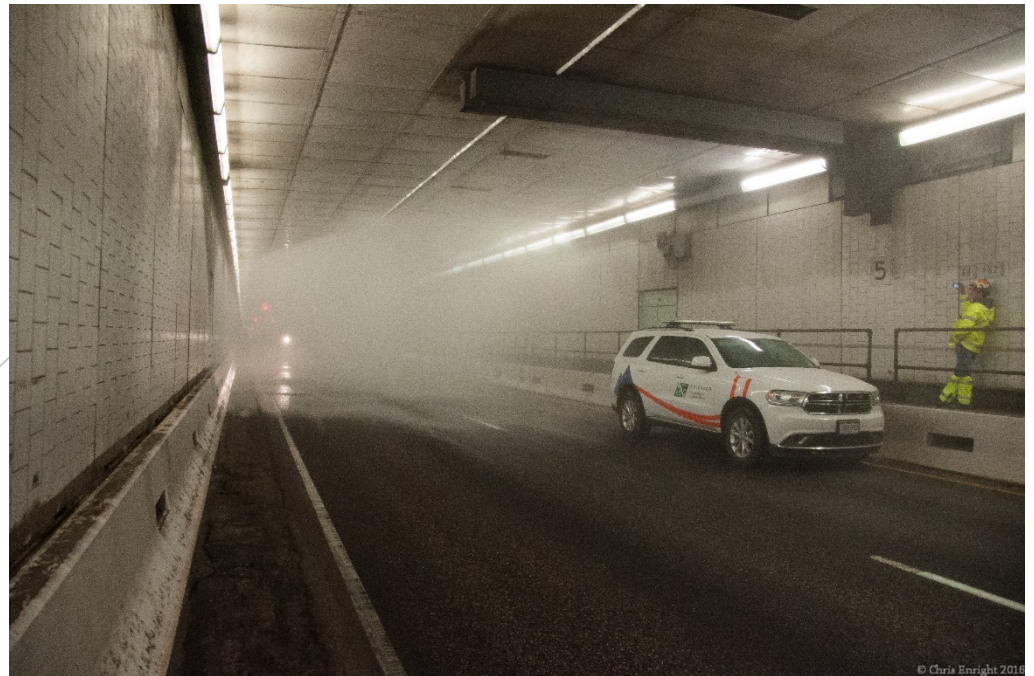
SPRINKLER OPERATION IN EISENHOWER TUNNEL
