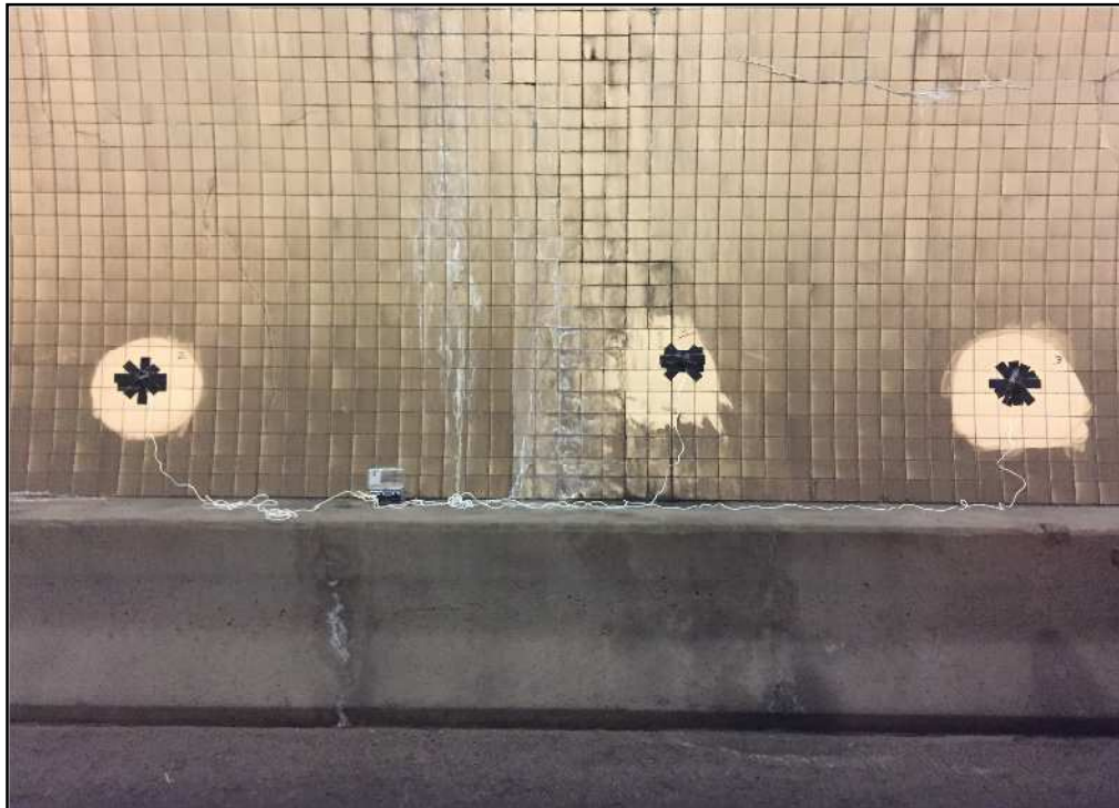
Figure 20: Example of logger installed at Hanging Lake Tunnel monitoring tile delamination with water and good tile surface on either side
