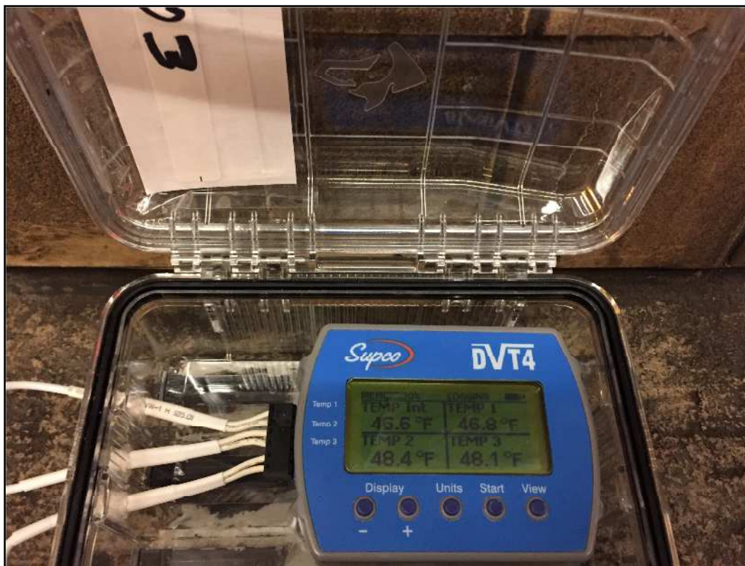
Figure 19: Thermocouple data logger installed in a custom waterproof box
