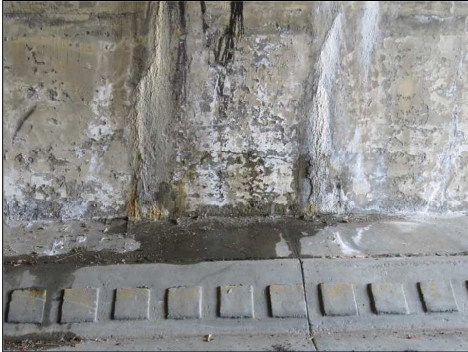
Figure 5: RGB image of area with pocket of water behind liner
