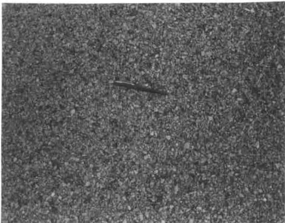
Photograph No. 8 4/28/82 Sections 2 & 6 -- RC-800 Rubberized binder. Typical appearance after 4 years.
