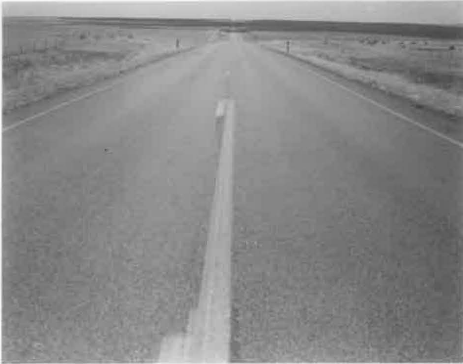
Photograph No. 13 4/28/82 Looking east at Test Sections 1-4 after 4 years. The performance of the different binders is difficult to distinguish without close inspection.
