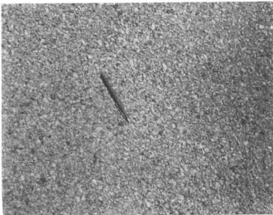
Photograph No. 10 4/28/82 Sections 3 & 7 — AC-10 binder. Typical appearance after 4 years.
