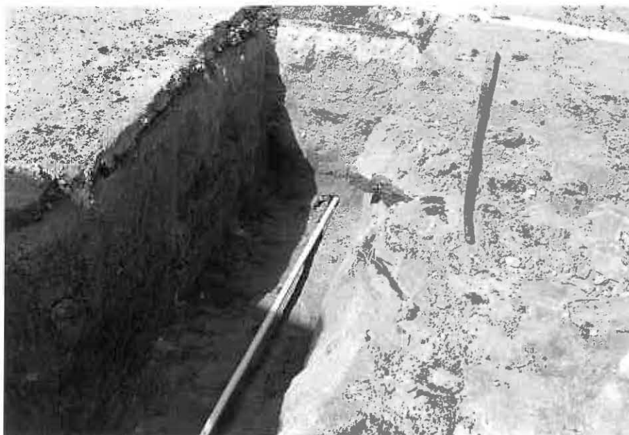
Photograph 5: The soil cell was inserted into the pilot hole under the outside edge of the driving lane.
