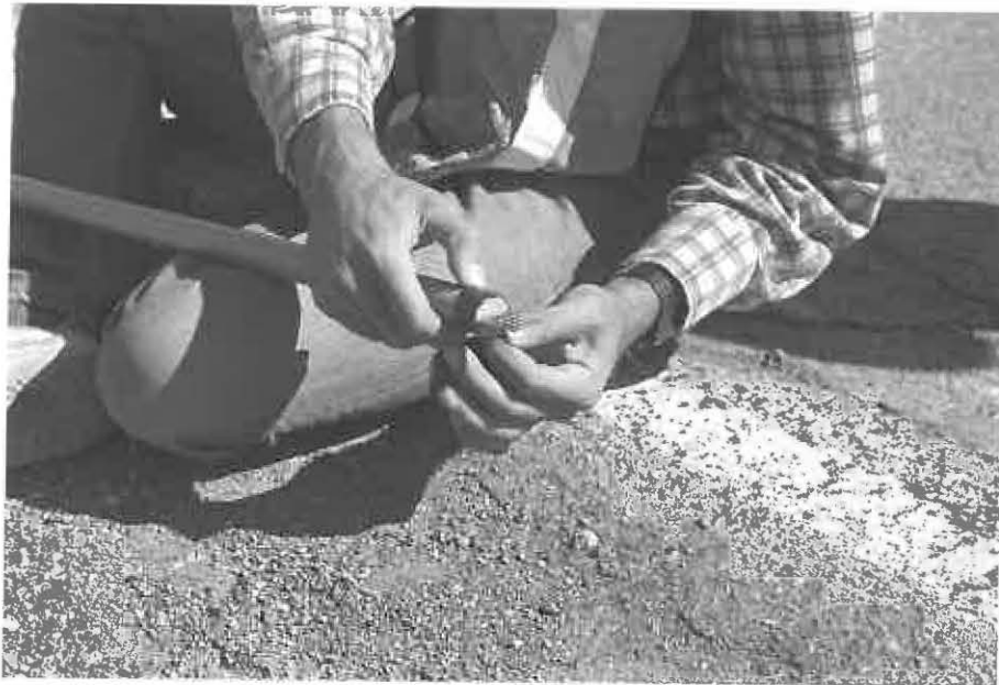
Photograph 4: One-inch PVC pipes were used to protect the lead wires from moisture and to secure the cell.
