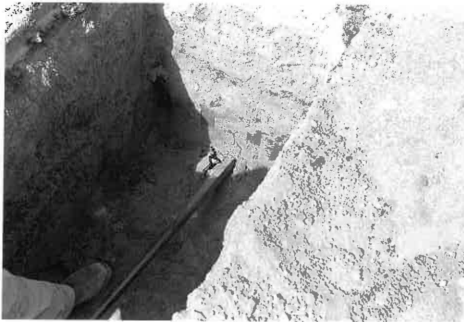
Photograph 3: A crow bar was used to provide a pilot hole for the soil cell.
