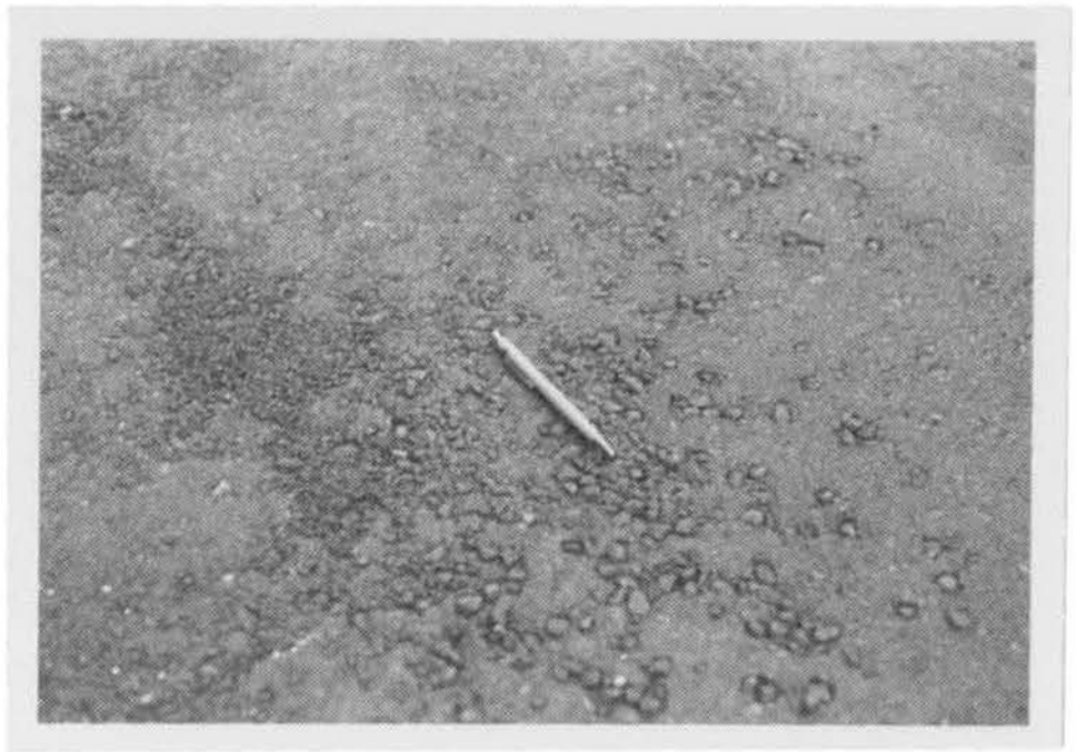
(J) Open surface area that was subsequently sealed
