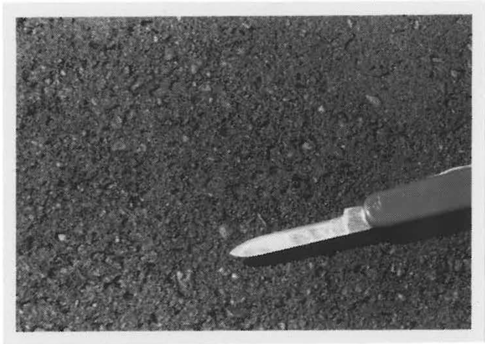
(K) Detail of pavement surface after the first rain
