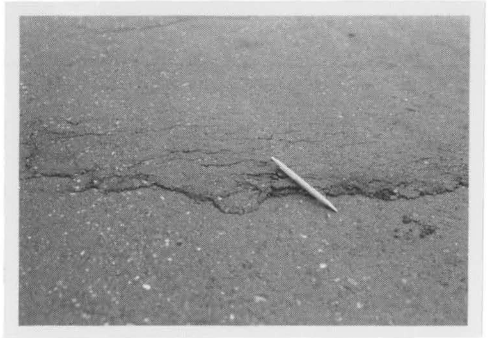
(I) An area of shoved pavement on the east side of the roadway
