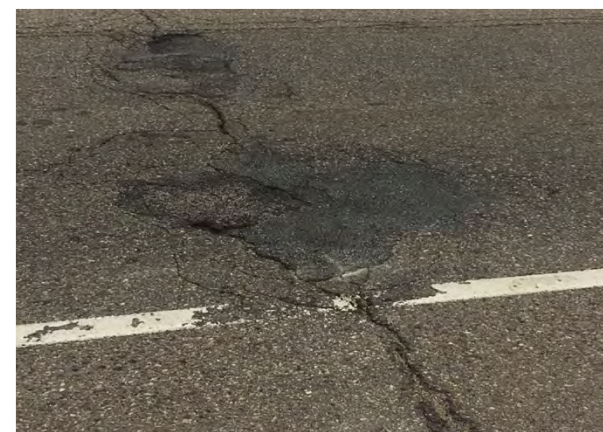
Poor pavement along a state highway
