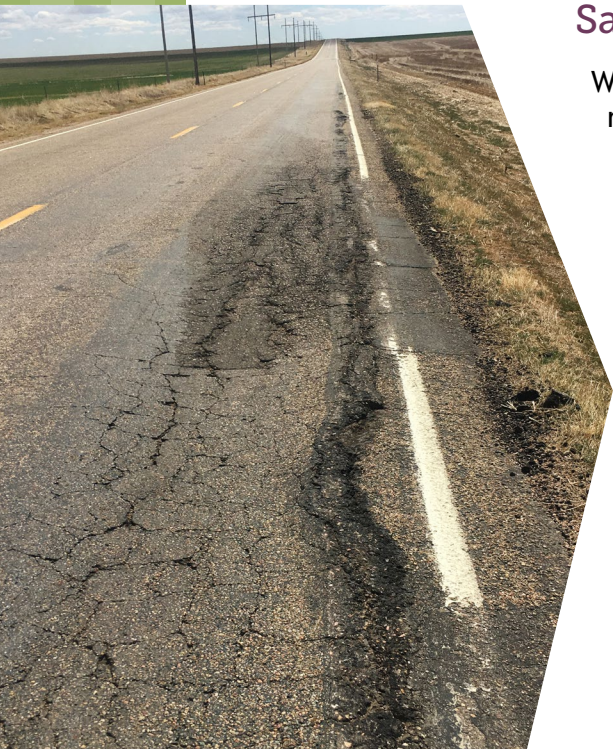
Pavement damage on US 385 in Cheyenne County
