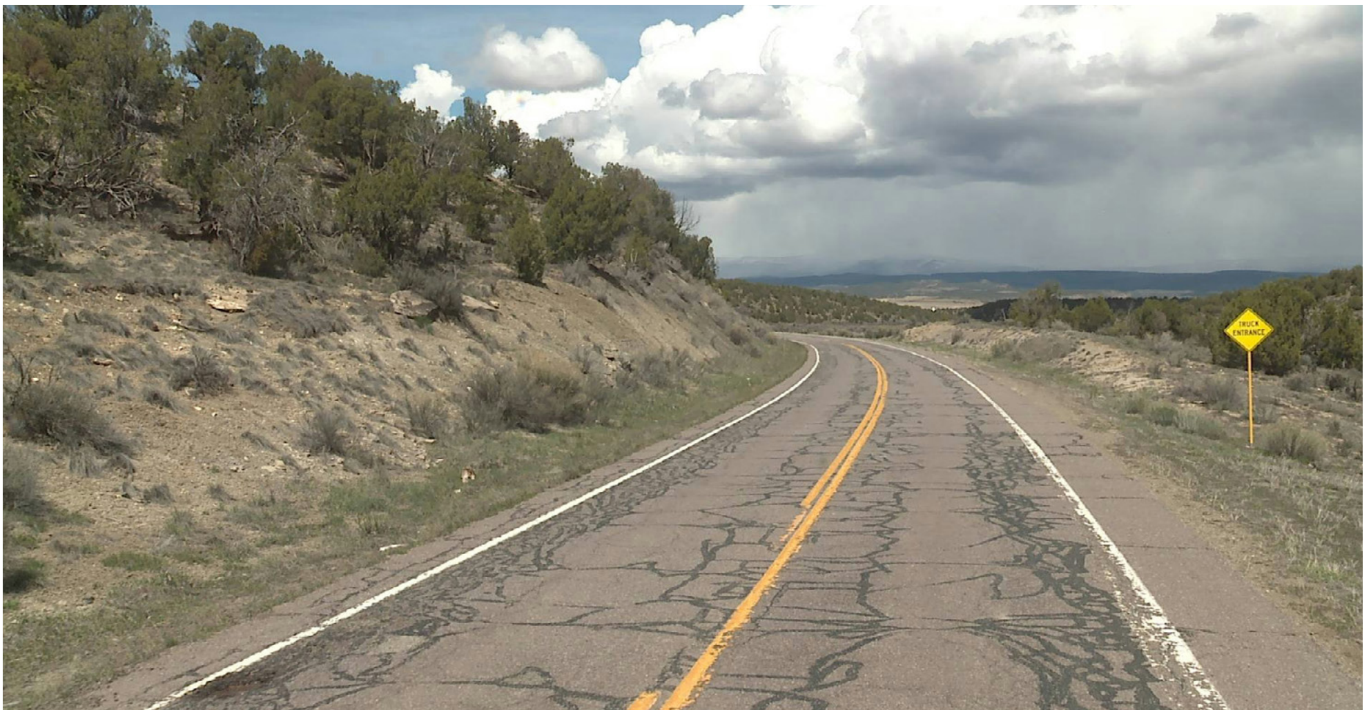
Poor pavement along a rural state highway
