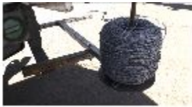
Fencing material is unspooled from the back of a truck, rather than unspooled by hand.
