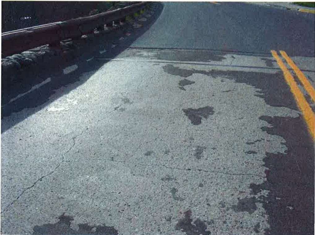
View Showing Cracks on Surface of Deck
