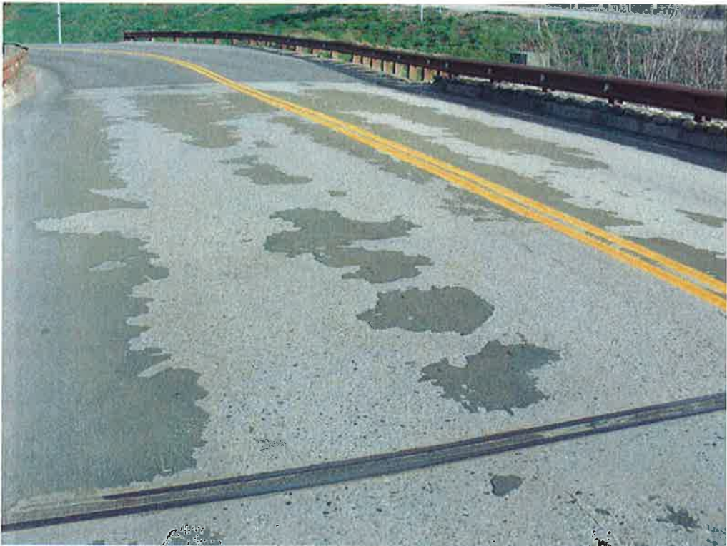
View Showing Polymer Coating Peeling Off of Deck Surface
