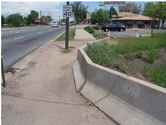
EXHIBIT 1-4: MISSING SIDEWALK SEGMENT SOUTH OF 12TH AVENUE
