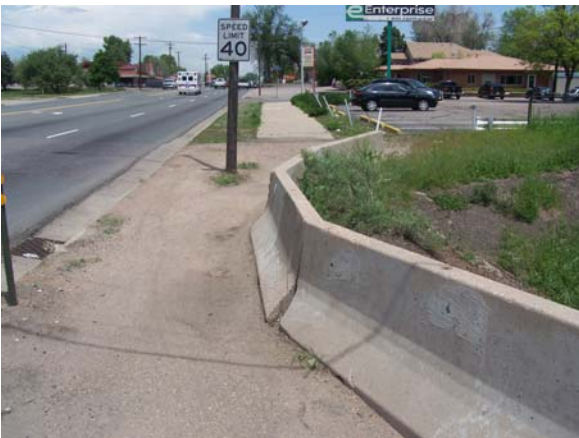
EXHIBIT 1-4: MISSING SIDEWALK SEGMENT SOUTH OF 12TH AVENUE
