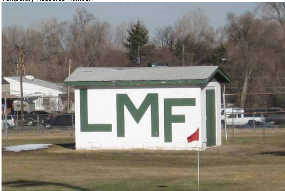
Photograph 35. Structure 12: Storage Outbuilding, west and south facades, view to the East, Northeast
