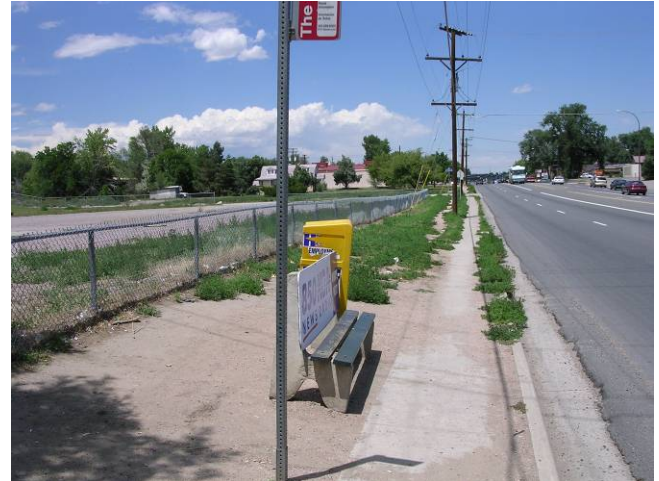
EXHIBIT 1-2: UTILITY POLES IN WALKWAY NEAR JEFFERSON COUNTY OPEN SCHOOL FORCE STUDENTS INTO TRAVEL LANES
